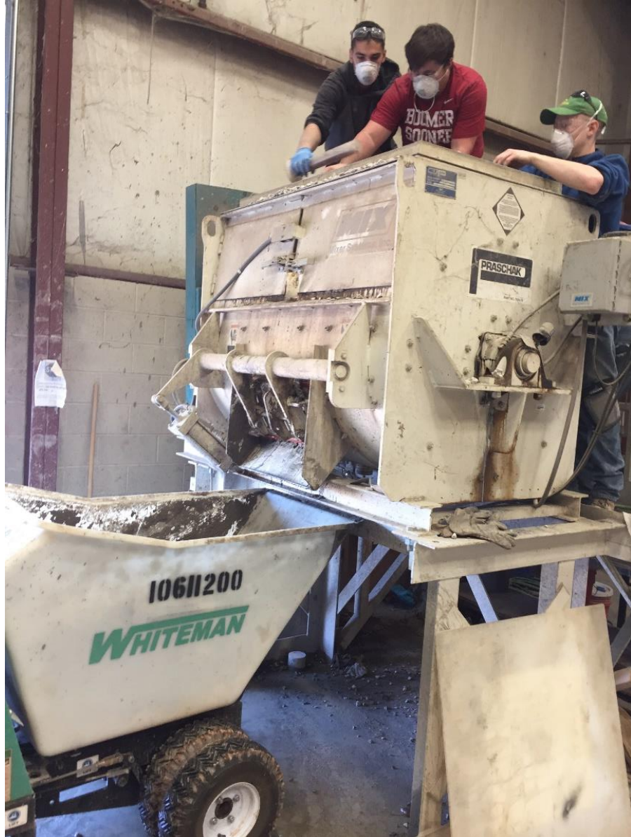
Figure 29, Concrete Mixer for Slabs
