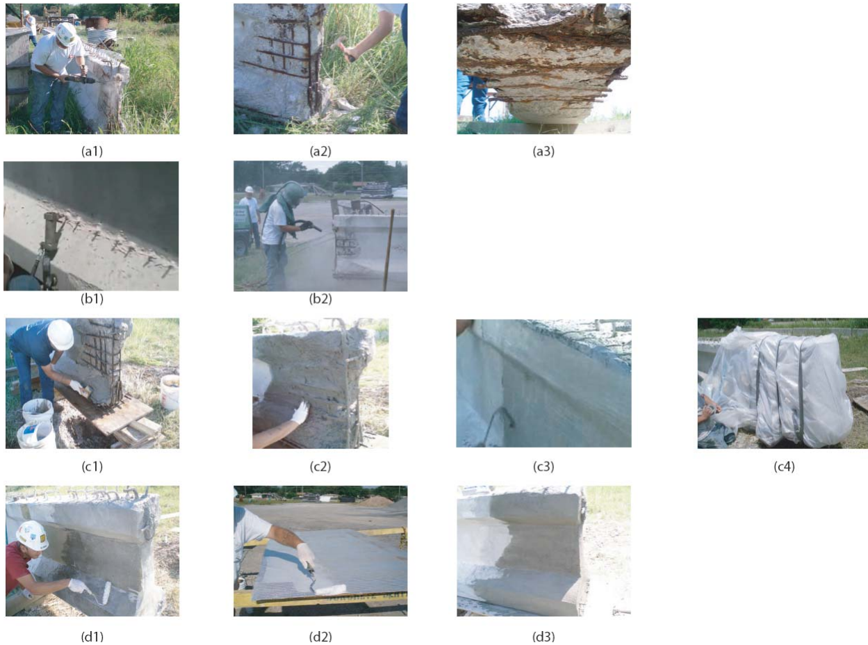
Figure 7: Retrofitting process documented by Mr. Christopher Davis: (a1) using a pneumatic drill to remove unsound concrete; (a2) using a standard hammer to remove unsound concrete so that more damage was not done; (a3) original view of damage to the bottom of the girder; (b1) sandblasting the surface; (b2) using a pressure injection epoxy to repair existing cracks; (c1) applying the initial coat of the wet mortar; (c2) applying the second coat of the intermediate mortar; (c3) the final mortar being the thickest and the repaired end finally shaped; (c4) the burlap sack that was used during curing; (d1) rolling on the epoxy to the girder prior to install the FRP wrap; (d2) impregnating the three-layer FRP wrap prior to installing it, and (d3) rolling the FRP wrap onto the girder to avoid air voids in the finished product.
