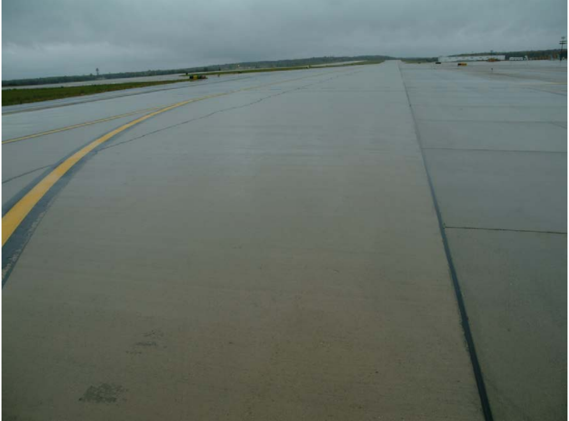
Figure 2: Airport Runway Slabs at Greater Rockford Airport (Ramseyer, 2018)
