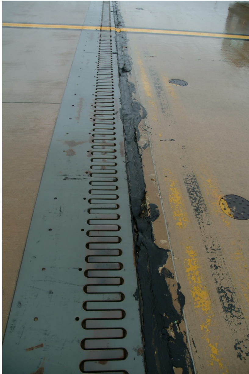
Figure 3: Separation of Post-Tensioned Slab from Expansion Joint at Greater Rockford Airport (Ramseyer, 2018)
