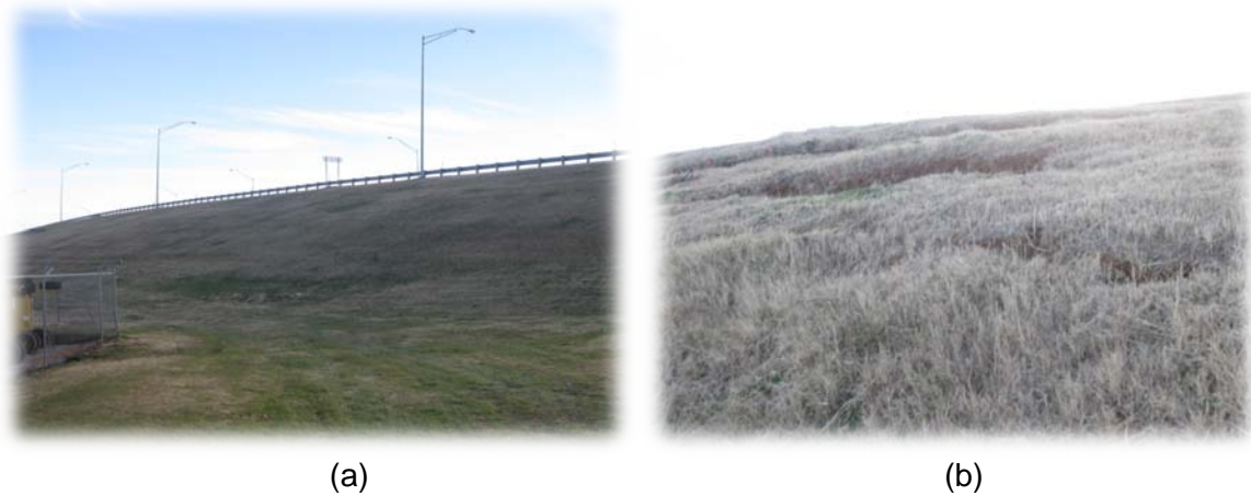
Figure 1. A failed slope of a highway embankment in Chickasha, OK
