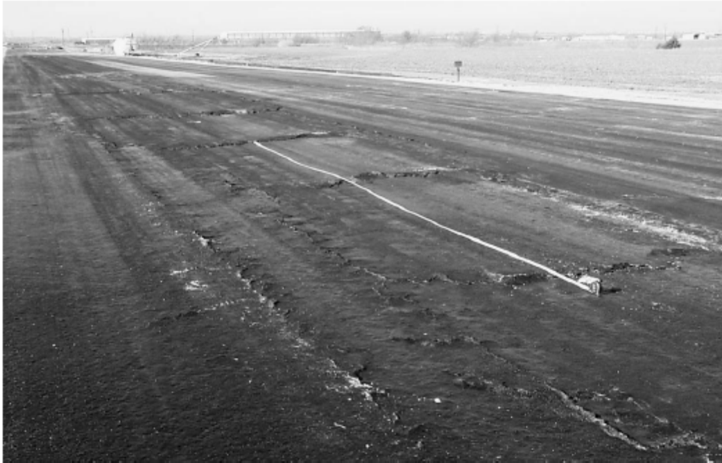
Figure 2-4. Sulfate Heave on U.S. 67 in Waxahachie, TX from Harris et al. 2003
