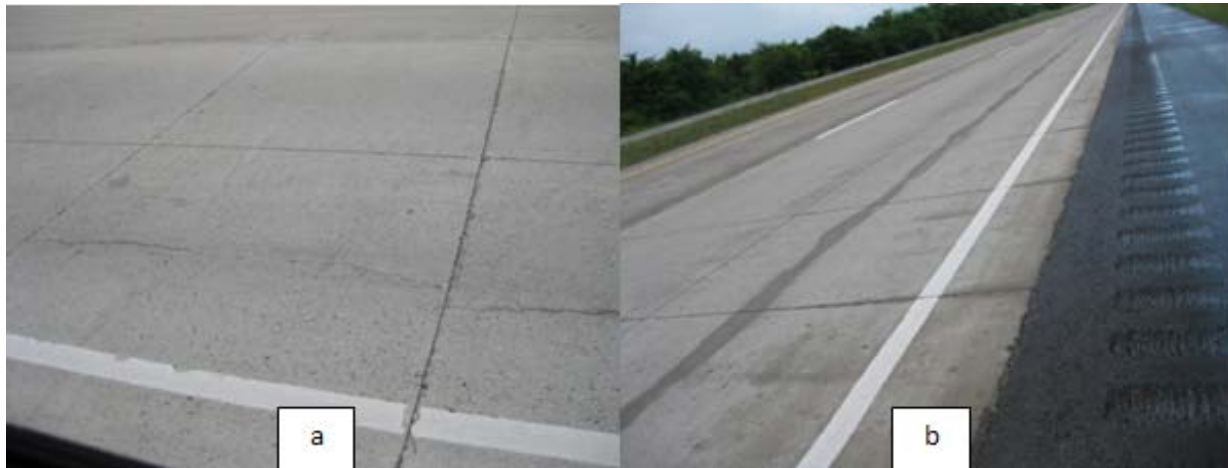
Figure 2.24 - Photo a showing the type of longitudinal cracking pattern. Photo b shows the cracks after heavy rains overnight. The seepage of water through the cracks is clearly visible.
