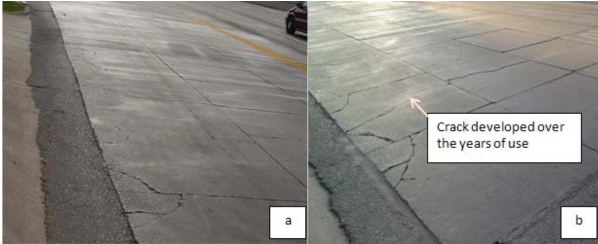
Figure 2.43 - Photos at the entrance to the gas station showing how the cracking has changed between 2004 and 2010. Photo a was taken in 2004 (David Cline, MacArthur Associated Consultants) and photo b is taken by the research team in 2010.
