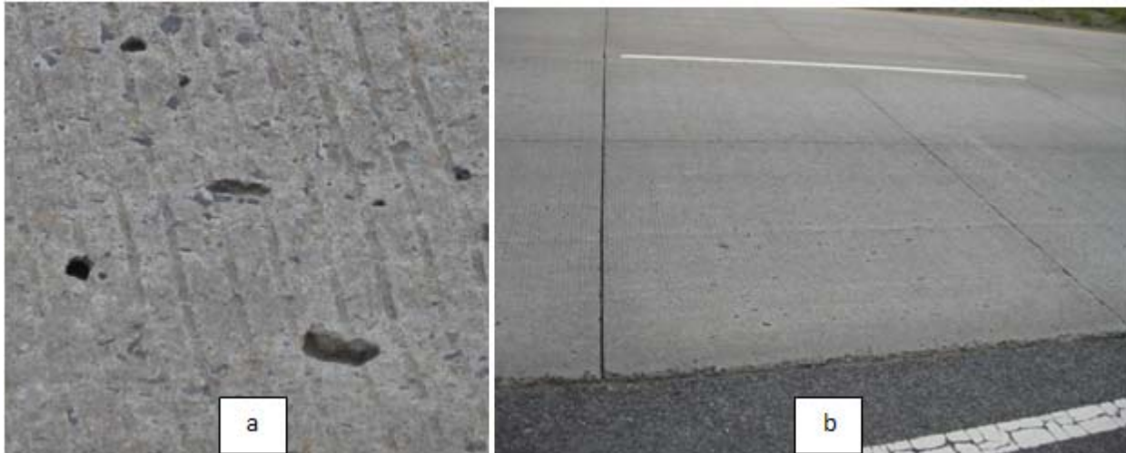
Figure 2.14 - Photo a showing pop outs (about 20 pop outs/panel) of larger aggregates (on about 24 panels) at about 0.5 miles from the south end of the overlay. Photo b is just the closer view of photo a.
