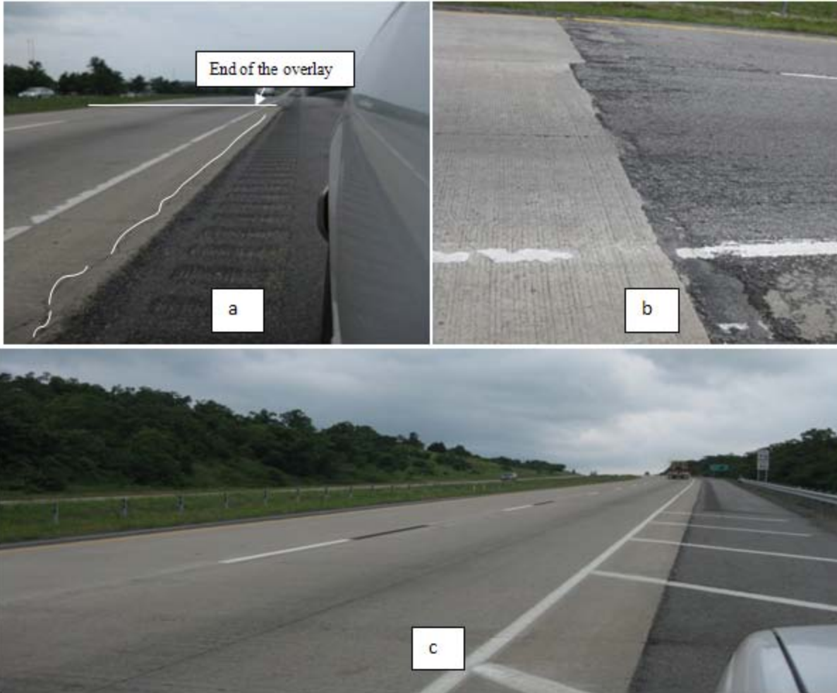
Figure 2.9 - Photo a shows the 13 panel long longitudinal crack at the end of the overlay. Photo b shows the transition of concrete into asphalt at the end of the overlay. Photo c shows overall good condition of the overlay.
