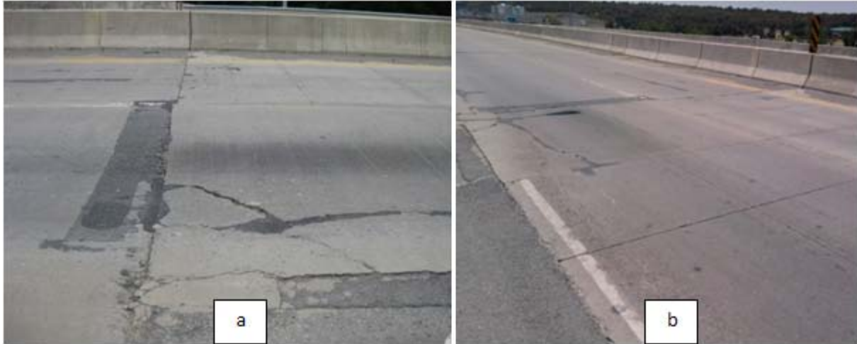
Figure 2.13 - Initial panels facing block cracking as shown in photo a. The first panel is replaced after initial failures with a full size panel as shown in photo b.
