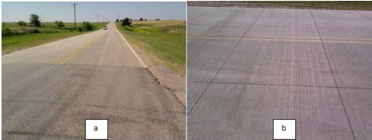
Figure 2.52 - North end of overlay. Photo a is taken looking towards south direction. Photo b is seven panel series from the end of the overlay.
