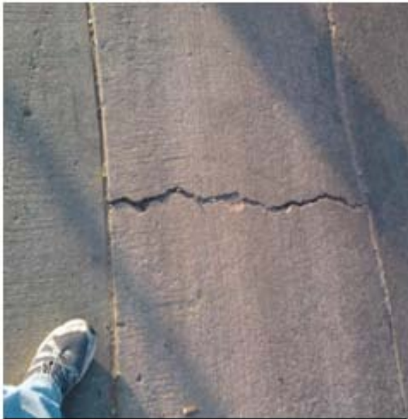
Figure 2.36 – Distress cracking in the shoulder.
