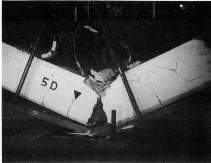
Figure C-5. Beam D-5 After Dynamic Load of 31.2 Kips
