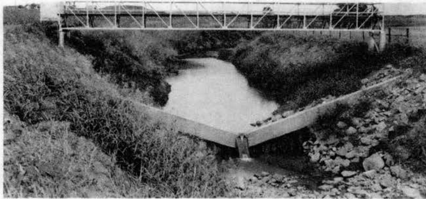
Figure 9. A typical weir control. This is the East Bitter Creek V-notch weir which has a slope of 3:1.
