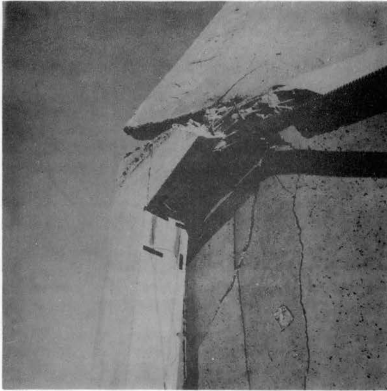
Figure 57. Torsional and bond failure near haunch
