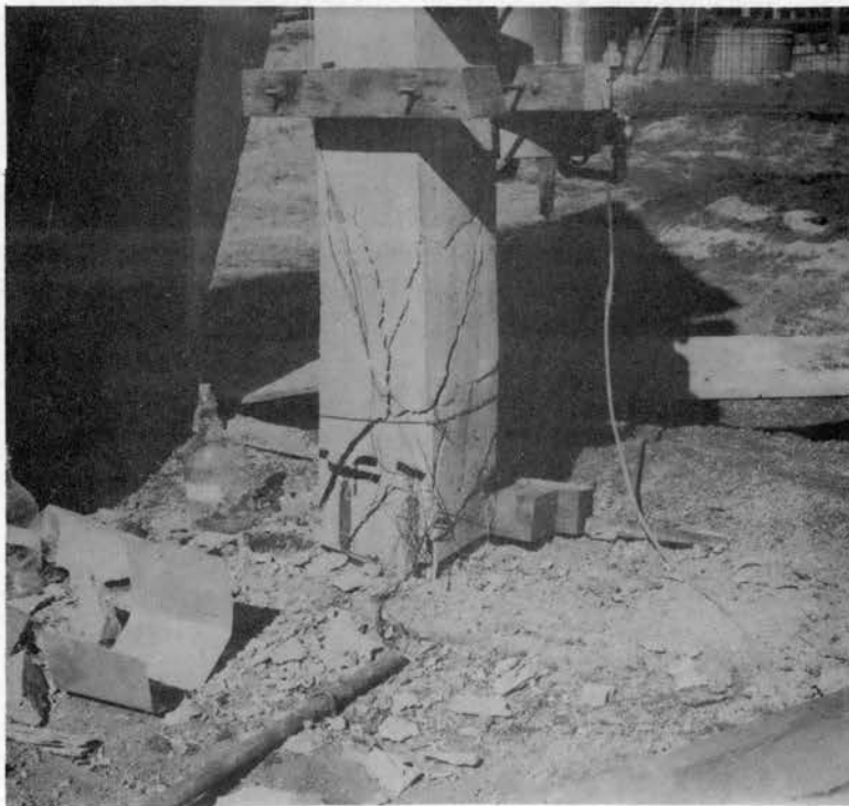
Figure 58. Failure of column EB
