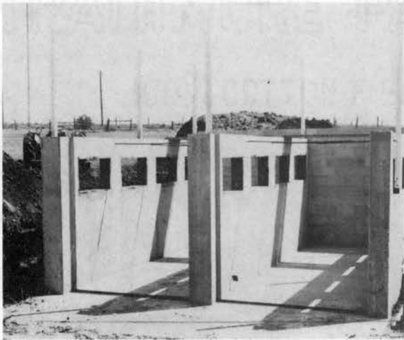
Figure 8. Waste collection tanks.
