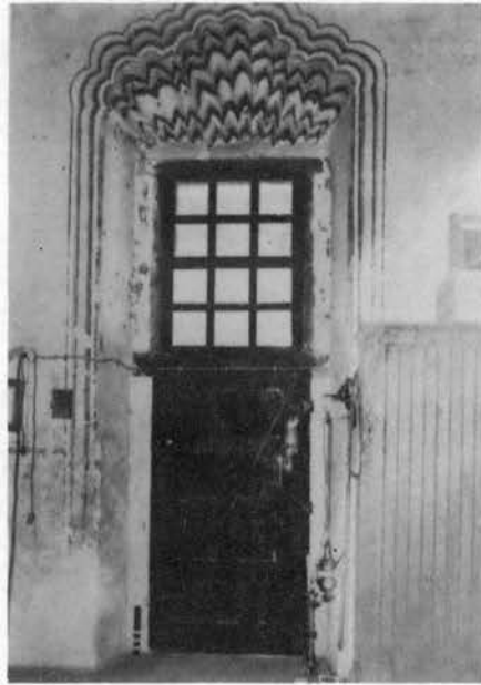
Figure 42. Door in the East Wall of the Sacristy Leading to the West Cloister, Showing the Shell. West Elevation.
