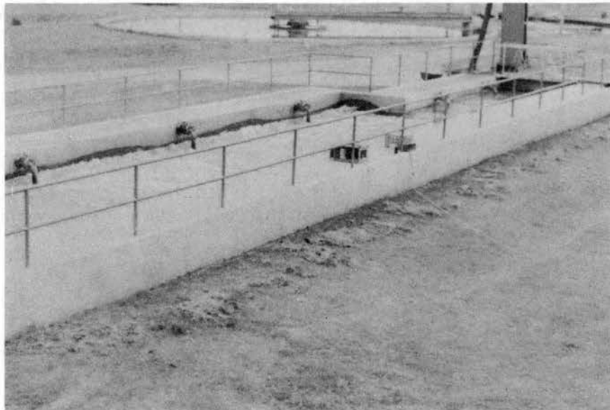
Figure 18 - Testing at pre-aeration tank.
