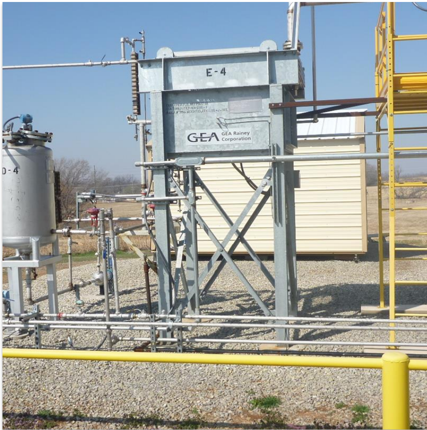
Air cooled condenser
