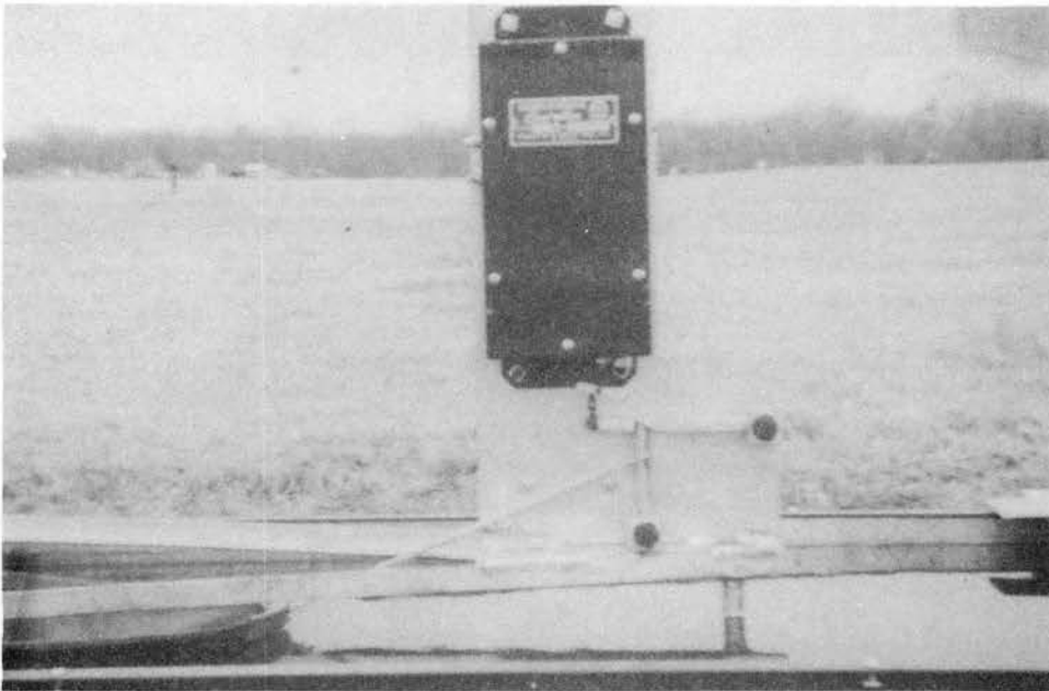
Figure 13. Time Operated Check Gate in Place
