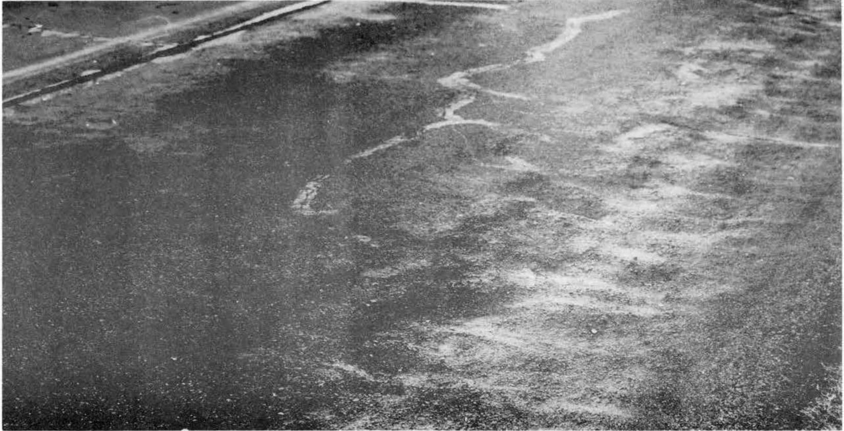
Figure 5.23. Shoulder Failure Because of Heavy Traffic
