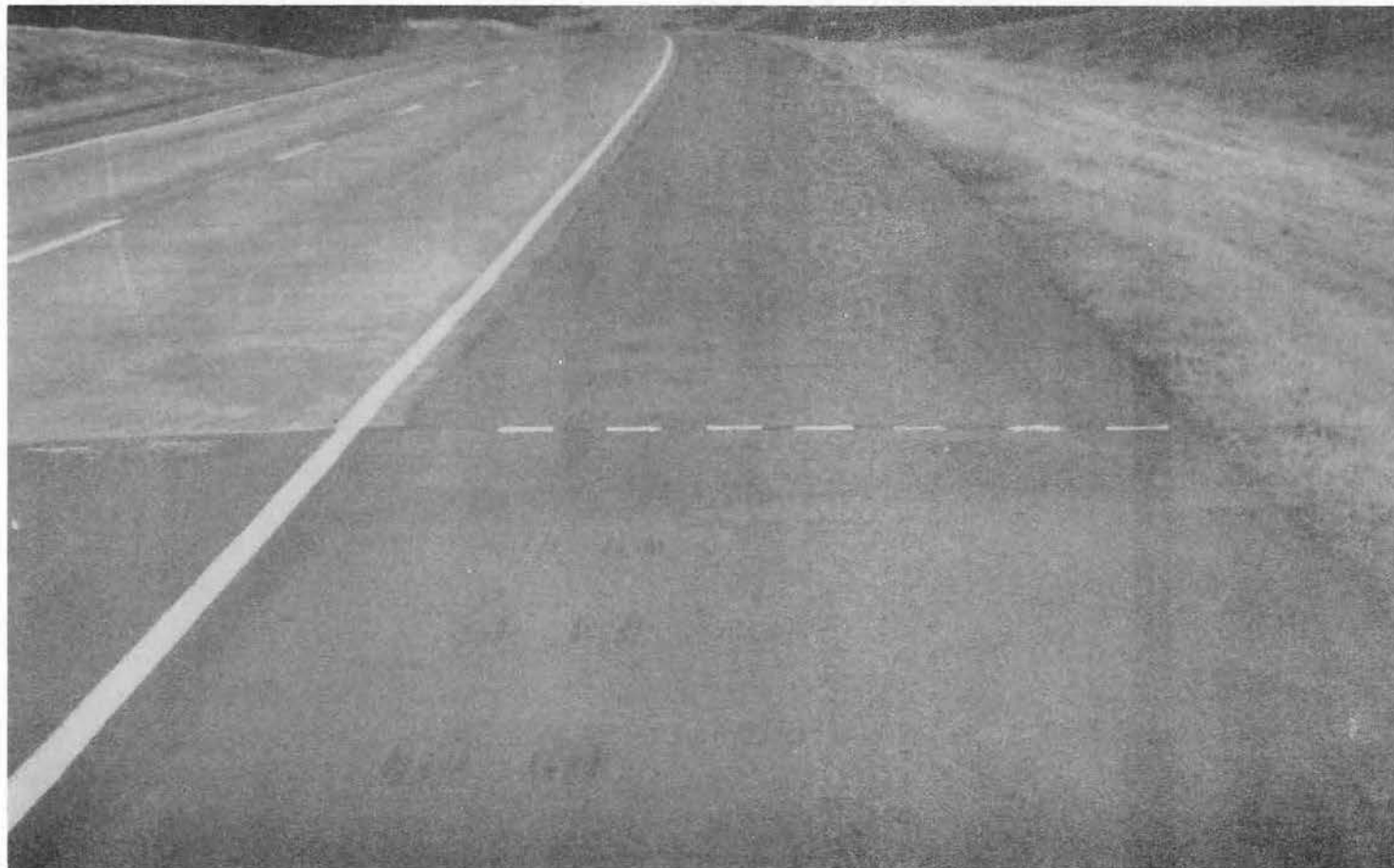
Figure 5.21. Shoulder Cracks Adjacent to Site Nos. 49 and 50
