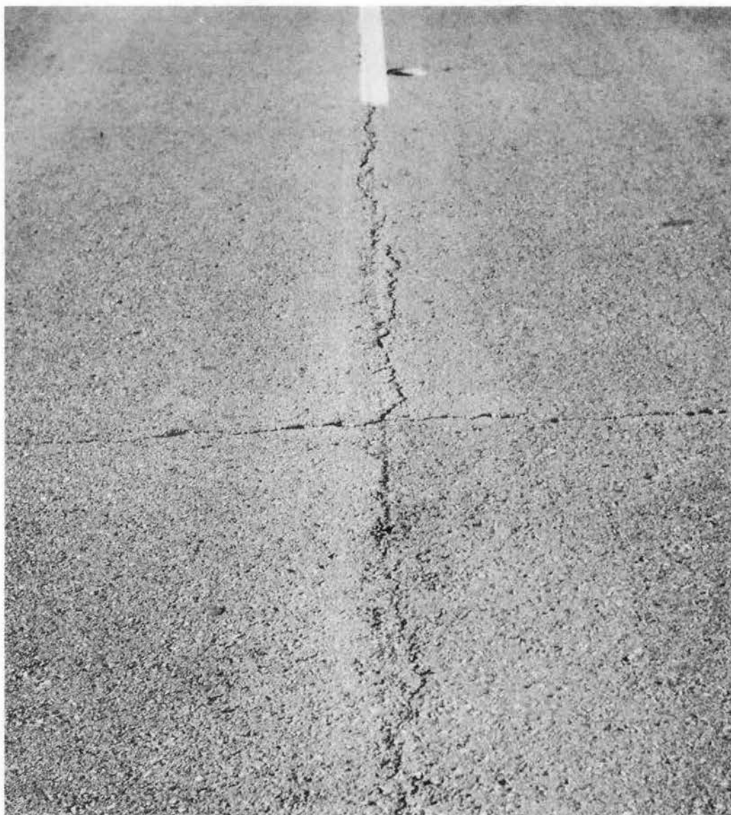
Figure 5.12. Transverse and Longitudinal Cracks in Overlay at Site No. 4
