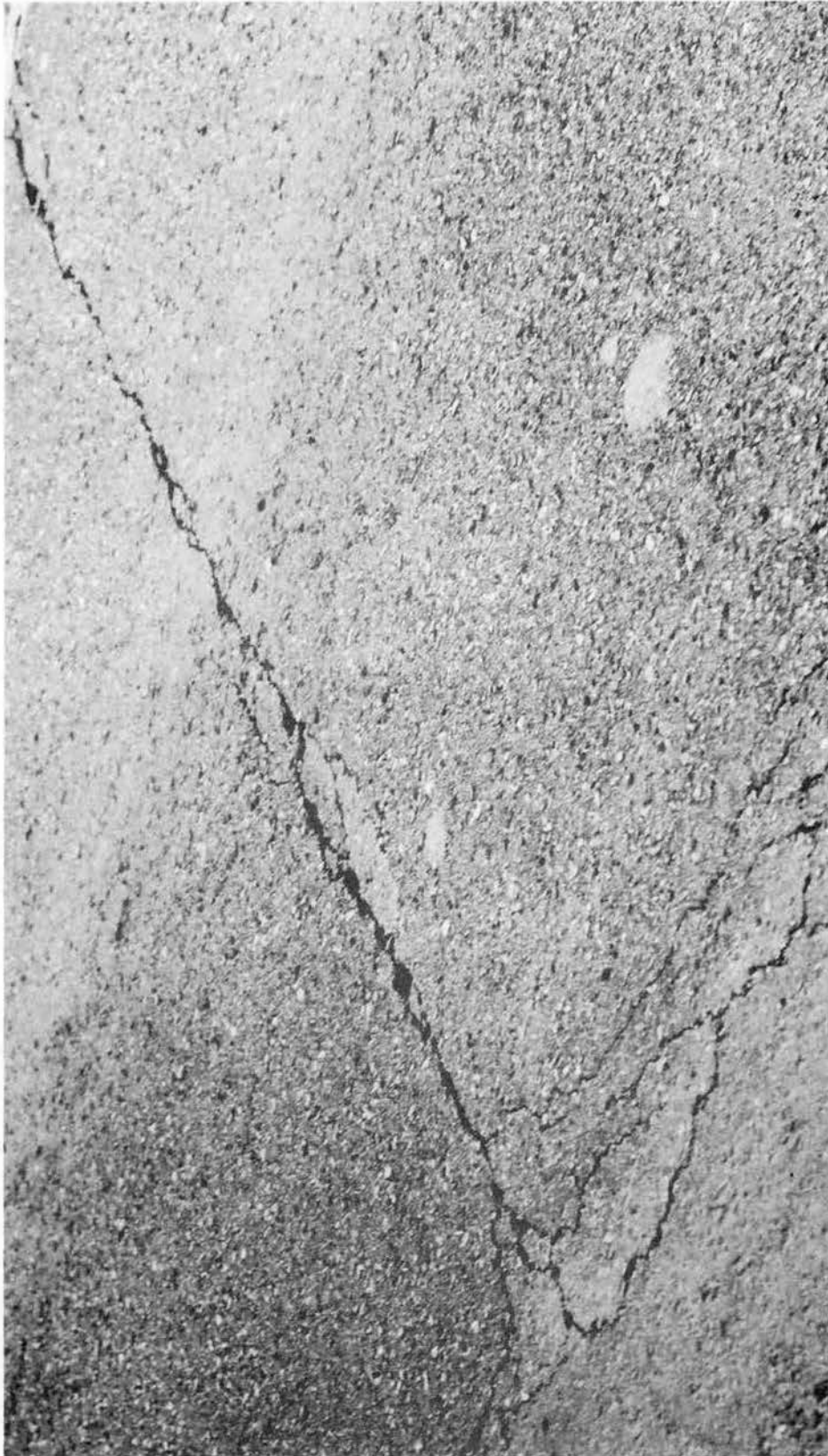
Figure 5.13. Close-up of Transverse and Longitudinal Crack Along Pavement Edge at Site No. 4
