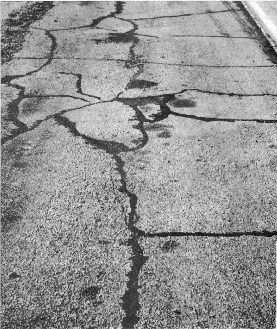
Figure 5.7. Transverse and Longitudinal Cracks in Outside Shoulder at Site No. 42
