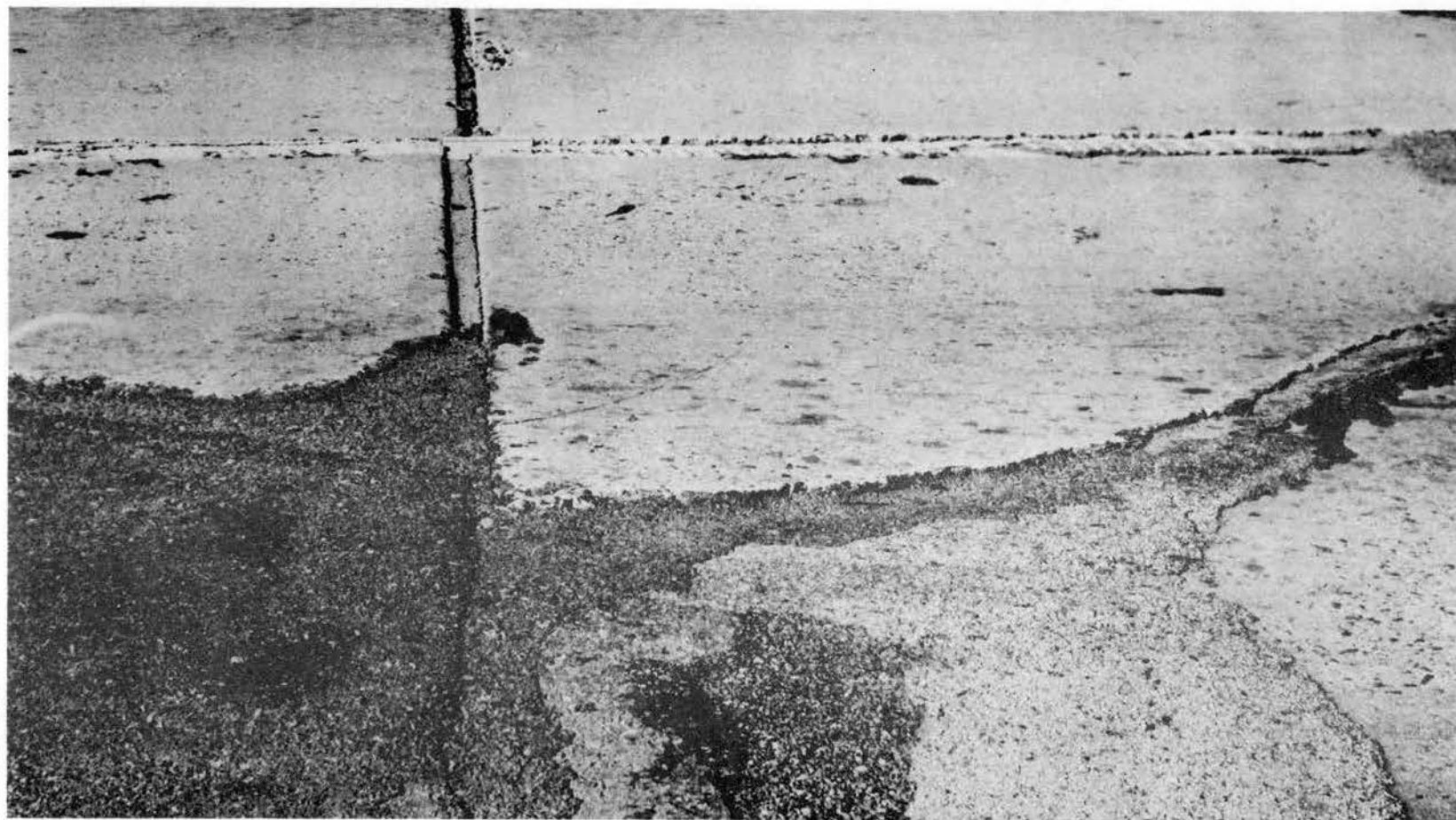
Figure 5.25. Close-up of Cracks and Joints in Figure 5.24
