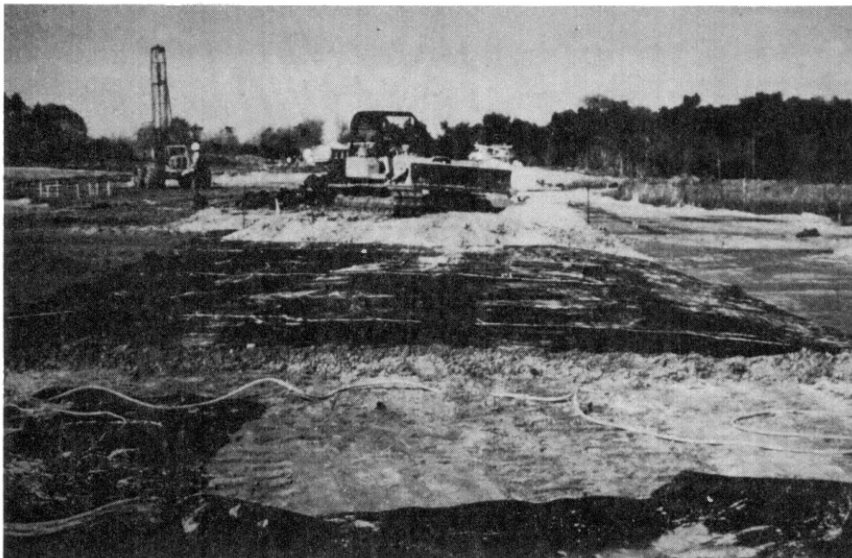
Figure 48. Fabric Folded Back into Toe of Structure to Serve as an Anchor to Prevent Fabric from Slipping
