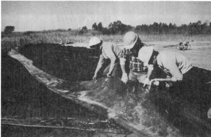
Figure 55. Nicolon 66475 Fabric Edge Being Sewn Together Prior to Folding the Newly Sewn Fabric Forward
