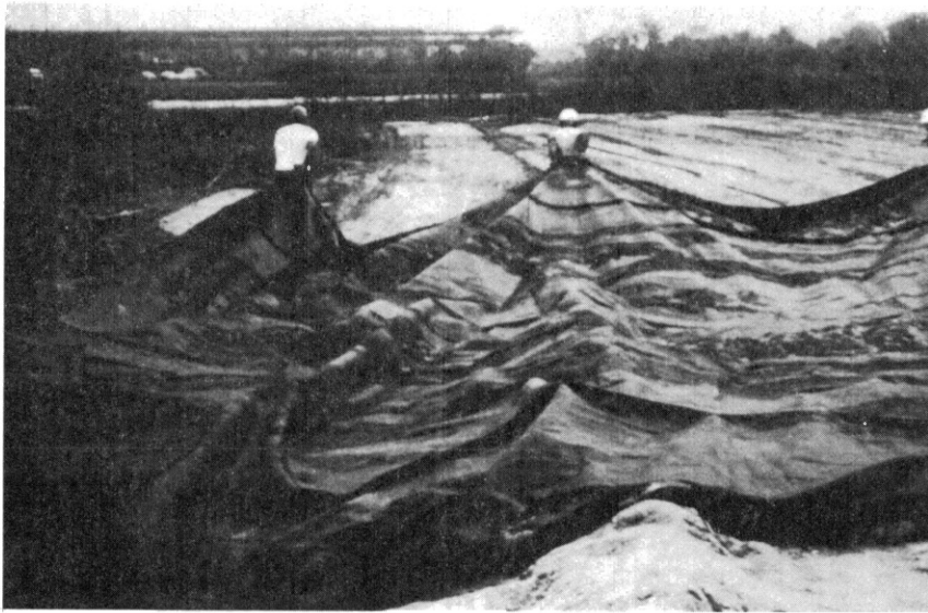
Figure 45. Advance Type I Fabric Being Placed, with Seams Perpendicular to Longitudinal Axis of Embankment, onto Sand Working Table
