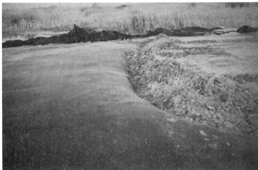
Figure 61. Fabric Being Stretched by Placement of Fill Material on Advancing Mud Wave Beneath the Fabric
