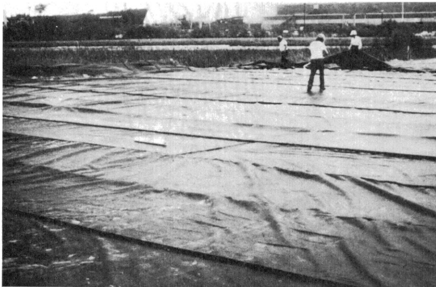
Figure 46. Placement of Advance Type I Fabric Prior to Placement of Fill Material
