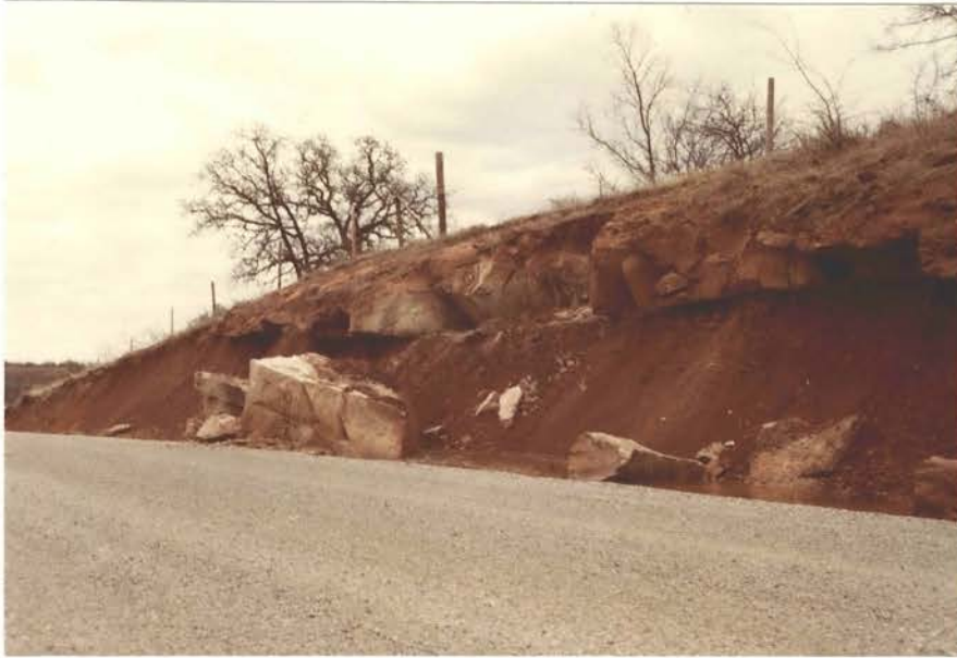
Figure 20. Rock fall along roadside near Arcadia, Oklahoma
