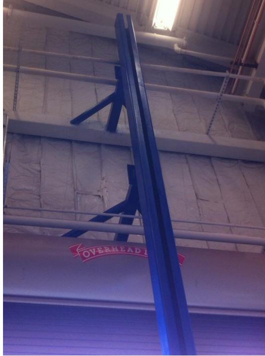
Figure 3.6: Top support (bracing) for the vertical beam
