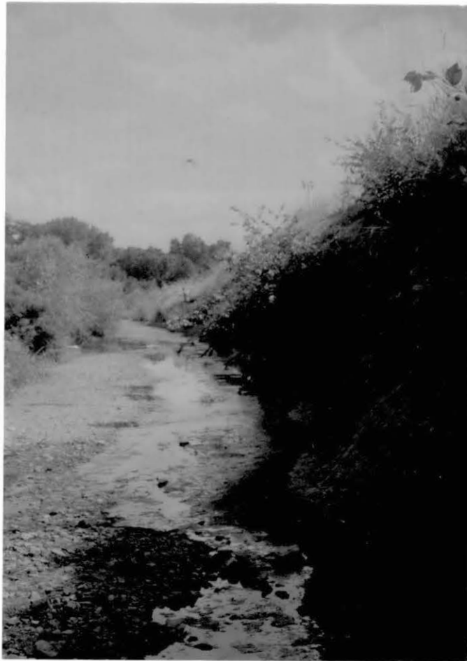
Figure 27. Man-made Channel Showing Seepage Zone Near Water Level
