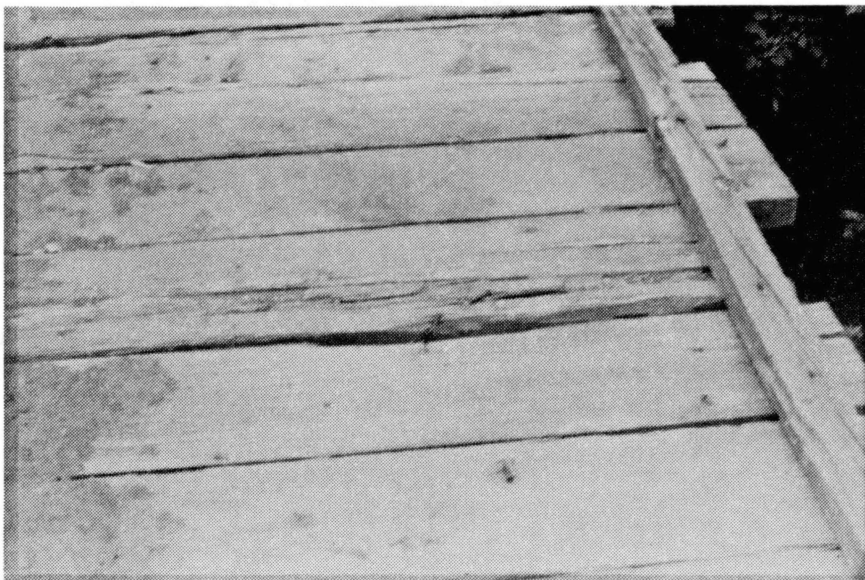
Figure 13. Timber Decking of Existing Bridge Showing Significant Weathering and Wear
