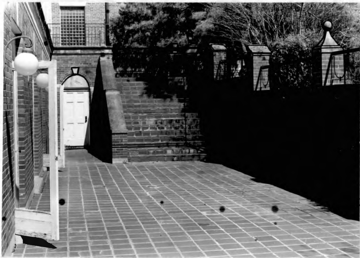
Figure 5. Modification of Basement Entrance to Eliminate Stairs on Ramp Side of East First Floor Entrance
