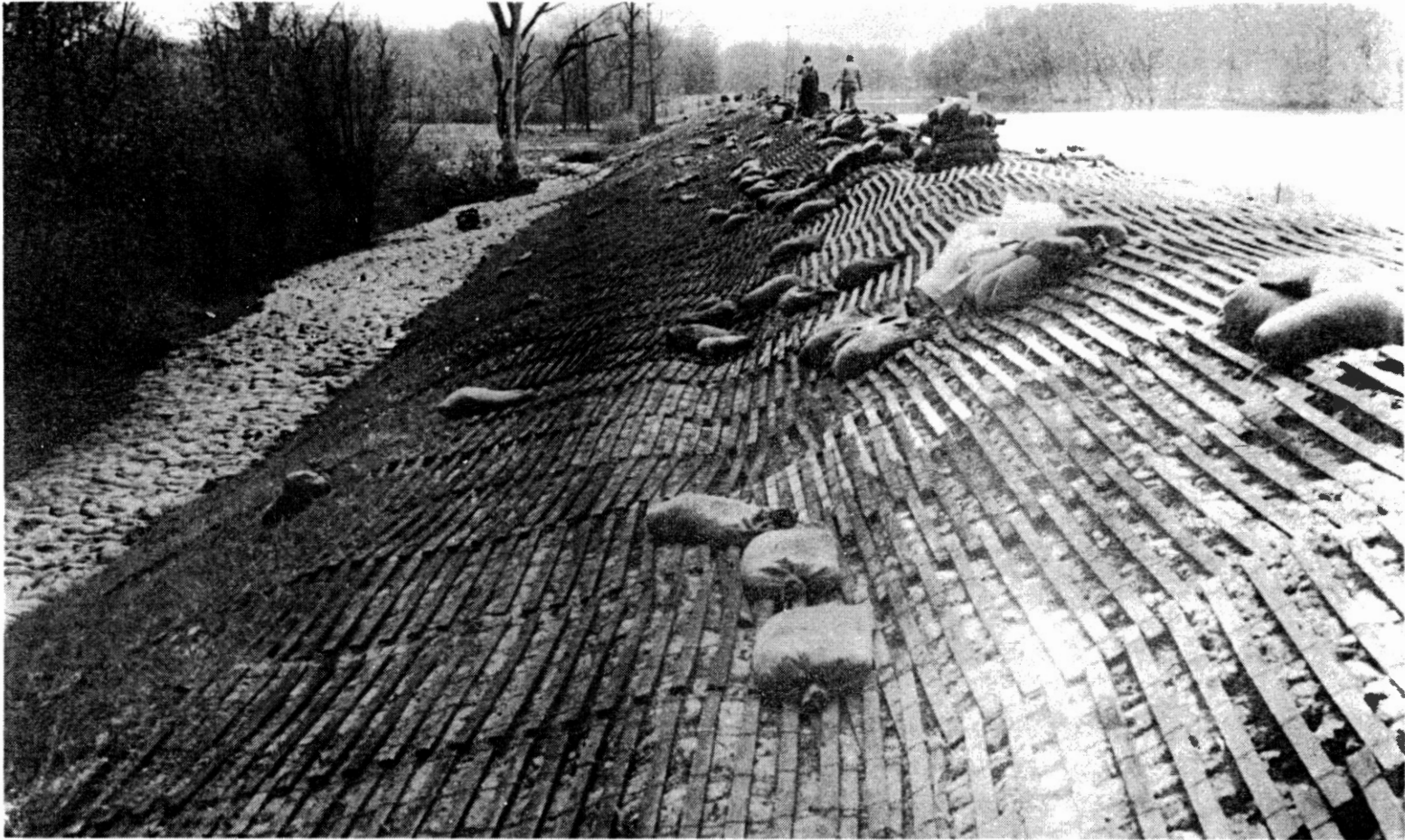
3 Figure 2 Unimproved Levee with Inadequate Through Seepage Control at Iowa River-Flint Creek Drainage District (May, 1965). (From U.S. Army Corps of Engineers, 1966).
