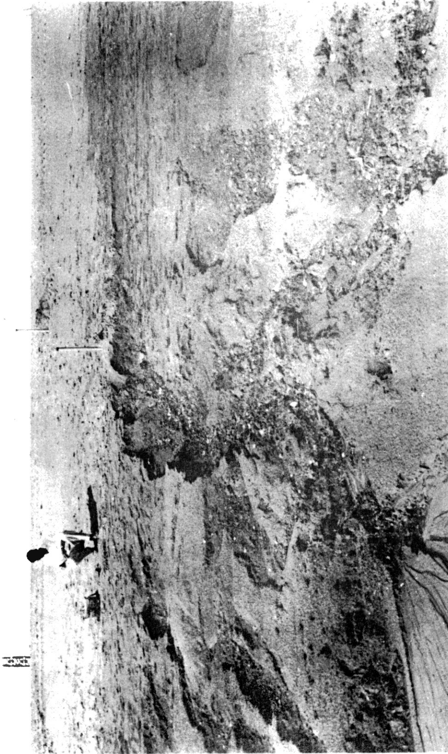
Figure 11 Landside Slope Erosion at Drury Test Section No. 2. (From U.S. Army Corps of Engineers, 1962).
