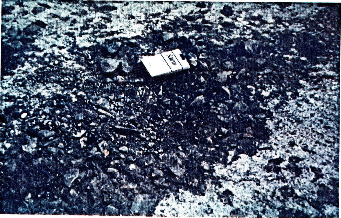
(a) Close-Up of Spalled Surface at a Cold Joint
