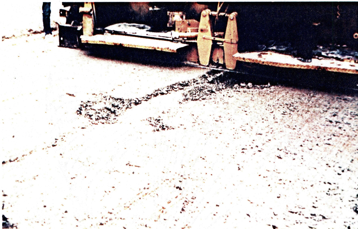
(a) Surface Tears Caused by Augers
