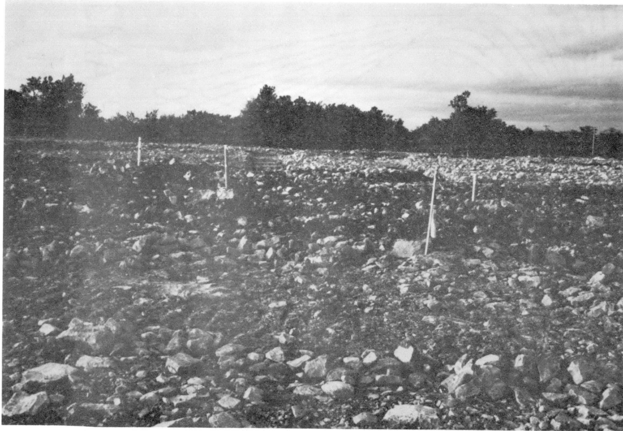
Figure 26. Photograph of Instrumentation at Test Section No. 2
