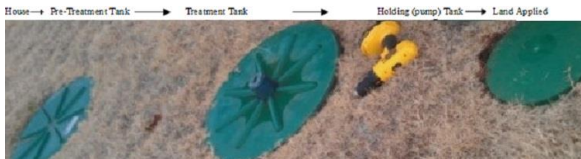
Figure 1. One of the three Aerobic Treatment Systems (ATS) where sample water was collected and tested for bacteria concentrations. The top of the tanks should be a minimum of 2 inches above the grounds surface; please note these tanks do not comply with that regulation (ODEQ, 2012).
