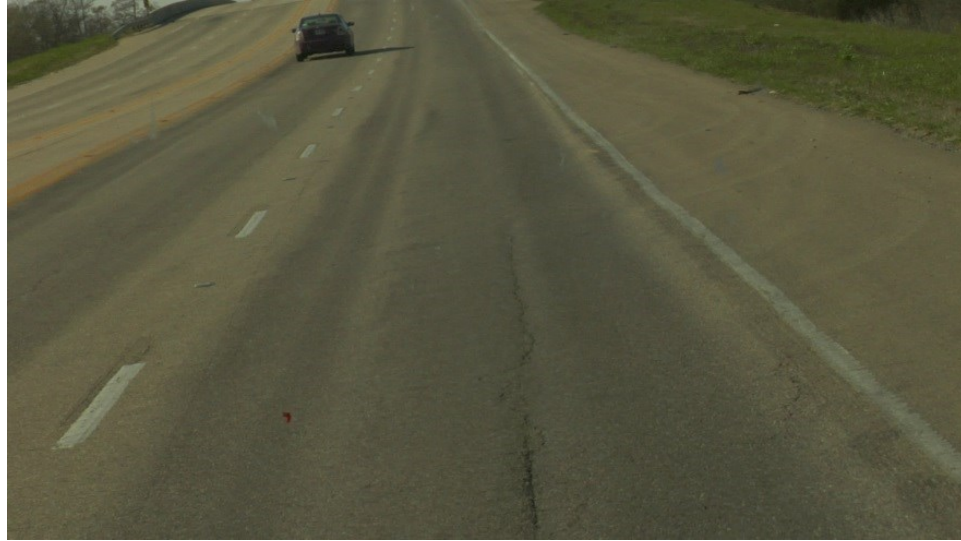
a. An Example of Pavement Rut on Highway
