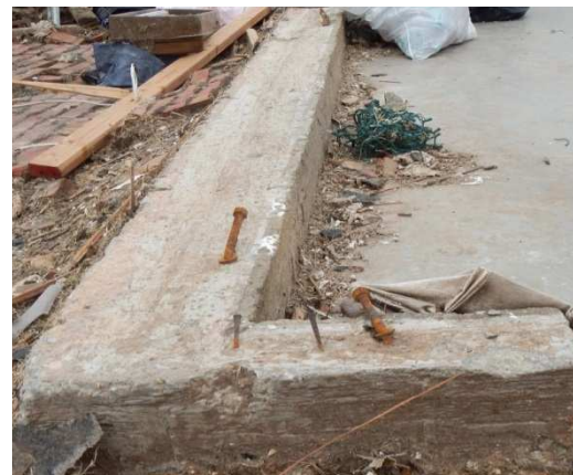
Figure 5: Failure of Bottom Plate
