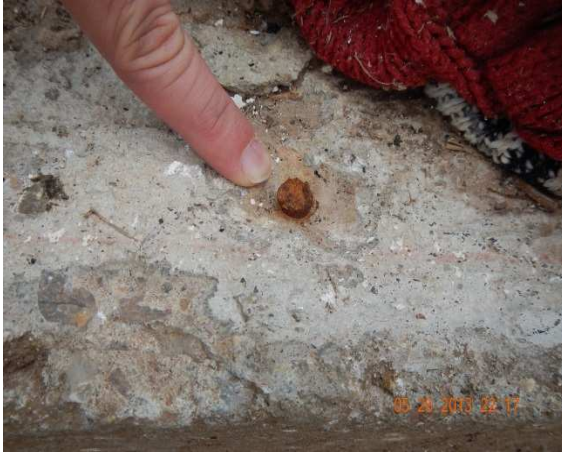
Figure 6: Shearing of Anchor Bolt
