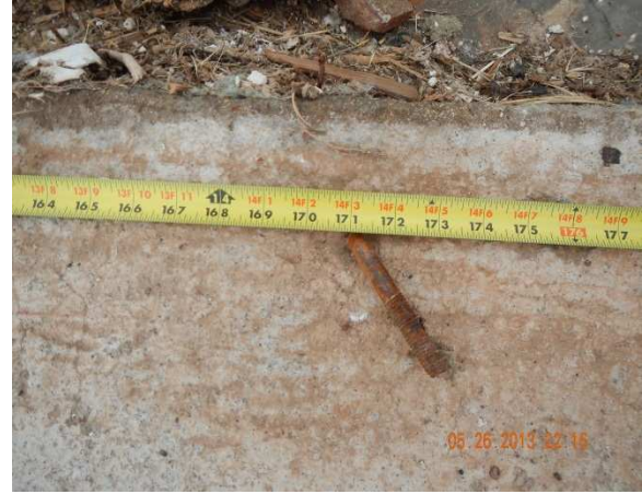
Figure 7: Failure of Bolt Thread
