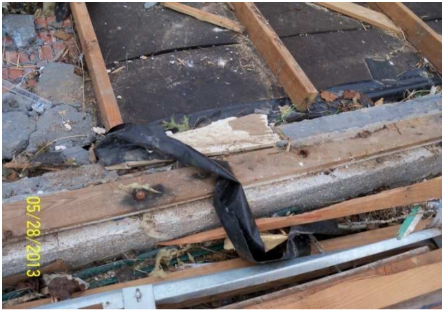
Figure 3: Failure of Stud to Bottom Plate Connection
