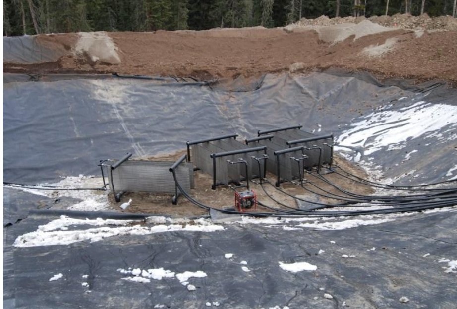
Figure 1.7: Plate heat exchanger arrays for home in Big Sky, MT. Reprinted, by permission, from Terry Proffer
