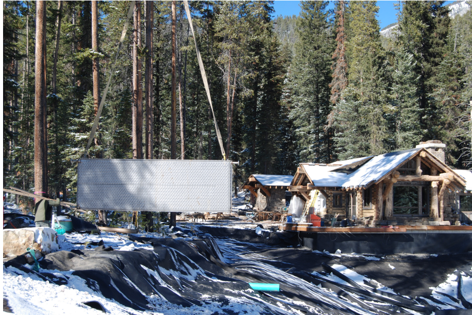
Figure 1.8: Plate heat exchanger array being lifted into place with a crane. Reprinted, by permission, from Terry Proffer
