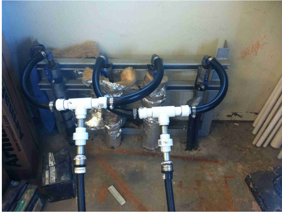
Figure 2.19: Ground heat exchanger connections where the water-water heat pump rejected/extracted excess heat energy
