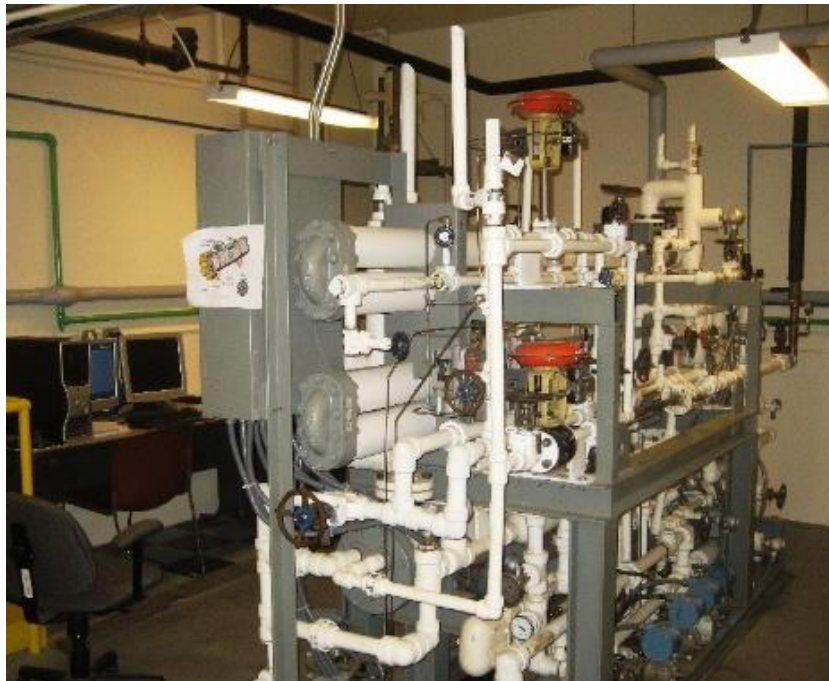
Figure 3-9: HX Network at Unit Operations Lab, OSU
