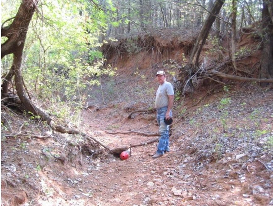
Figure 19 Sediment trap installation in a dry stream channel in the Bull Creek watershed.
