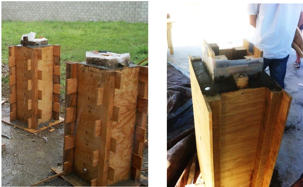
Figure 15: Outer Molds (Jigsaw Cut on Left, Flat Cut on Right) with Inner Mold and Curing Concrete
