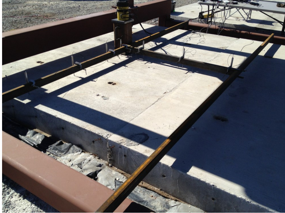
Figure 49 Instrumentation set for Test Location 1. Note that this test is located at the center of Panel A.
