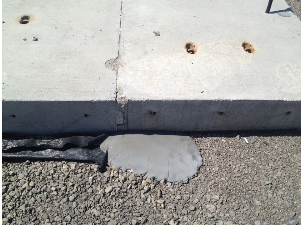
Figure 42 Leaking grout at the joint of panel II-B2 and II-C
