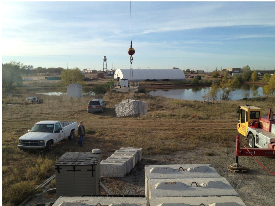
Figure 46 Concrete blocks being lifted for placement on top of the test frame
