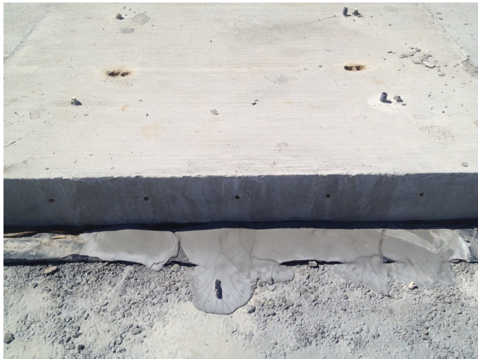
Figure 41 Leaking grout at the middle of panel I-B1
