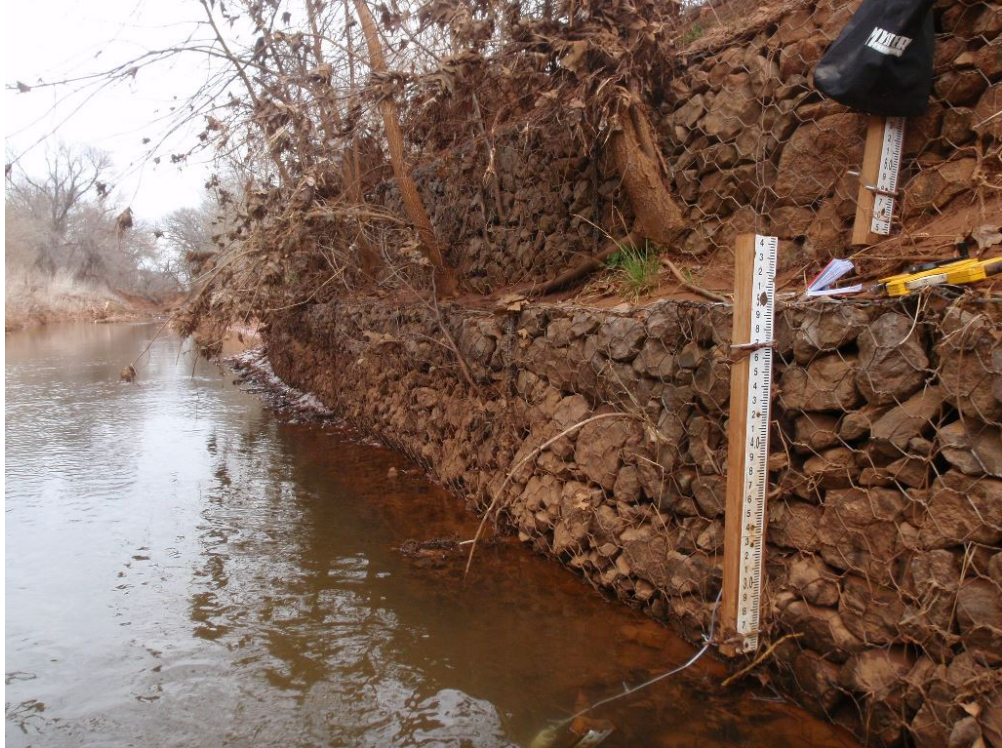
Figure A.1.2: Little River at 60 th Ave NE HOBOT initial installation.
