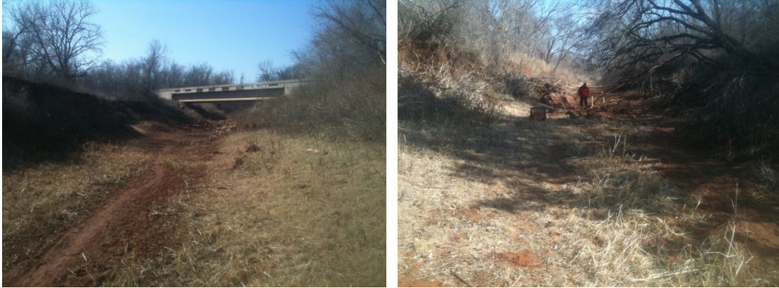
Figure F.20.1: FGM Site DBC-01 – Cross Section - Looking upstream (lt); Looking downstream (rt).
