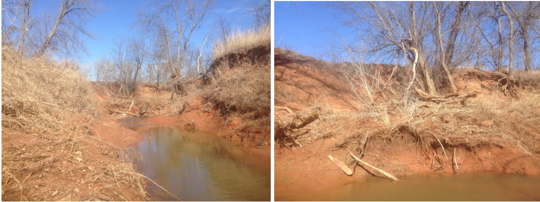
Figure F.7.7: FGM Site LR-07 – Bank 3–Facing downstream (lt); Bank 4-Bank (rt).
