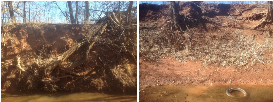
Figure F.8.2: FGM Site LR-08 – Cross Section - Left Bank (lt) – Right bank (rt).
