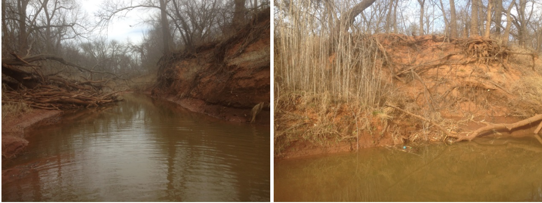
Figure F.6.4: FGM Site LR-06 – Bank 1-Facing downstream (lt); Bank 2-Bank (rt).
