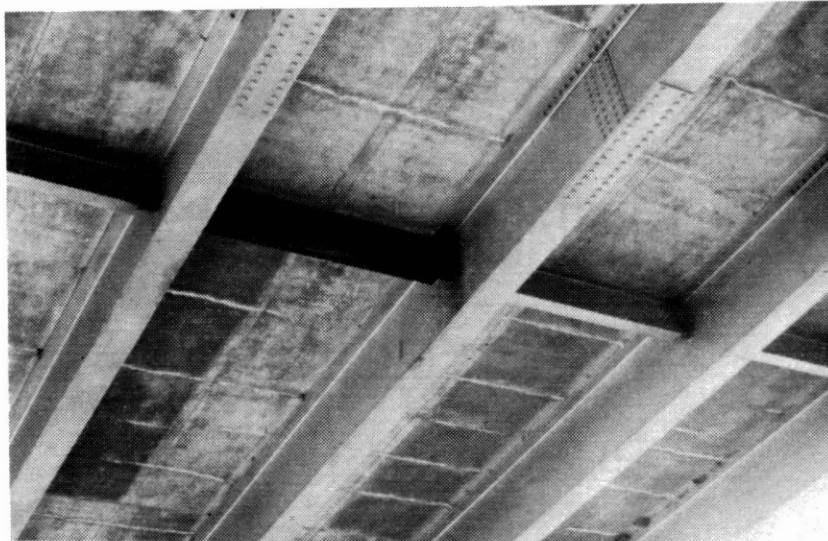
Figure 2. Placement of Diaphragms
