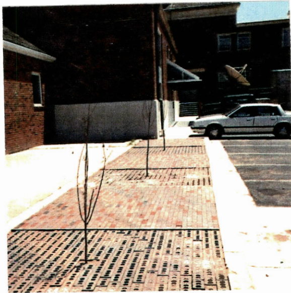
Figure 20. Vet. Med. Lot 66 Perimeter Condition, Spring 1988.
