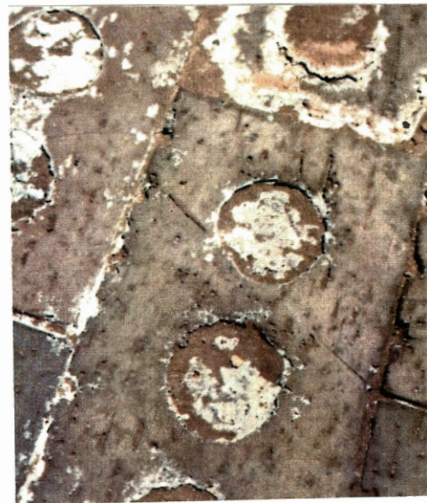
Figure 21. Vet. Med. Lot 66 Close Up of Gray Substance on Brick.
