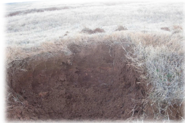
Figure 3.1. Excavation pit where soil samples were taken from the failed slope in Chickasha, OK
