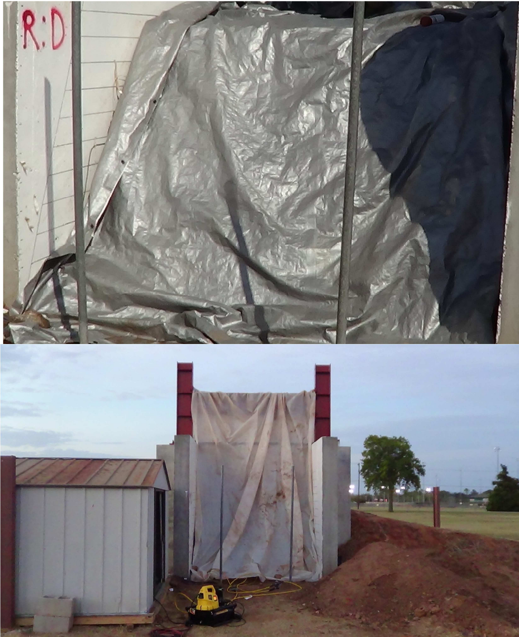
Figure 5.7. Covering the embankment with tarp and plastic sheet to avoid losing moisture content and reach moisture equilibrium
