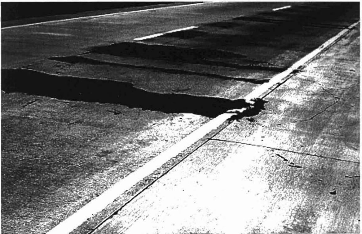
Figure A56. Patches on F-219(35) southbound.
