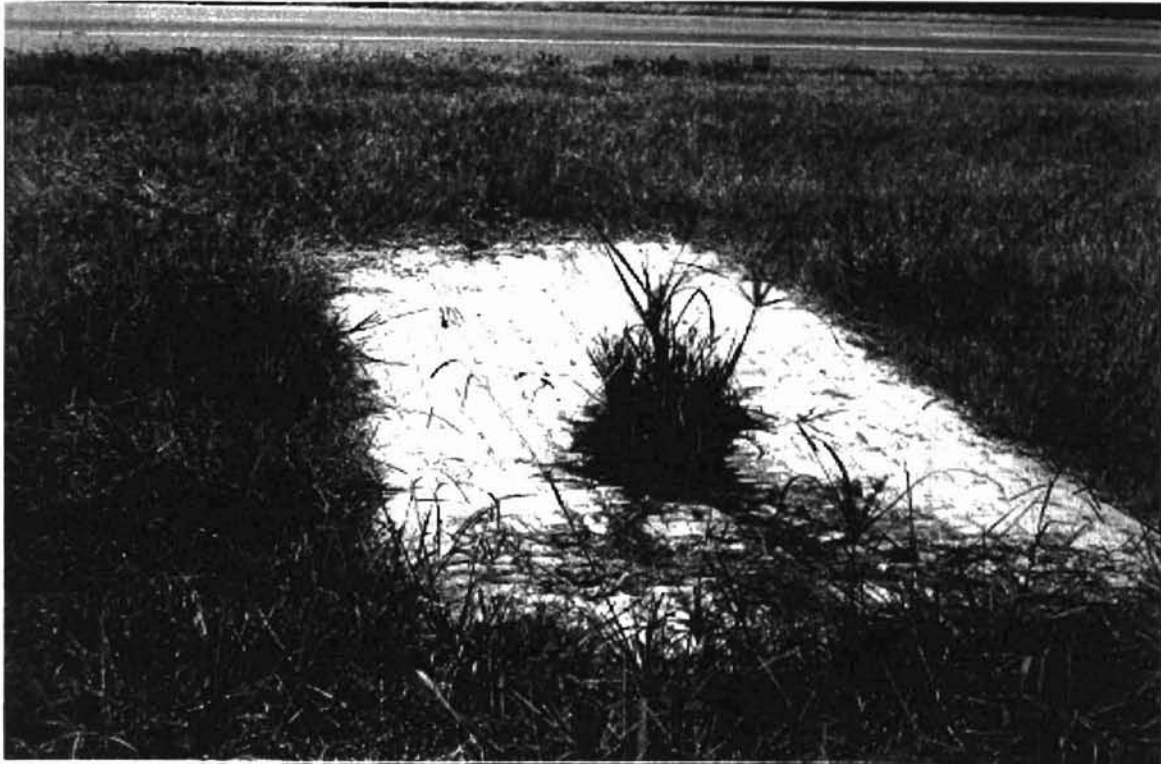
Figure A25. Outlet of pavement underdrain
