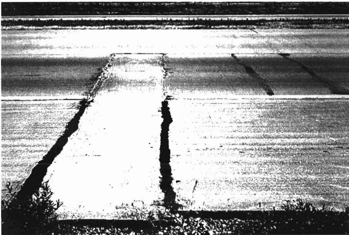
Fig. A76. Repair of punchout. Drain constructed to increase drainage under pavement.
