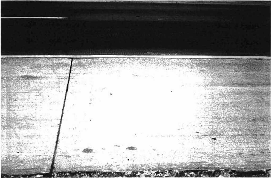
Figure A52. Typical condition of shoulder and pavement of F-299(99) northbound.
