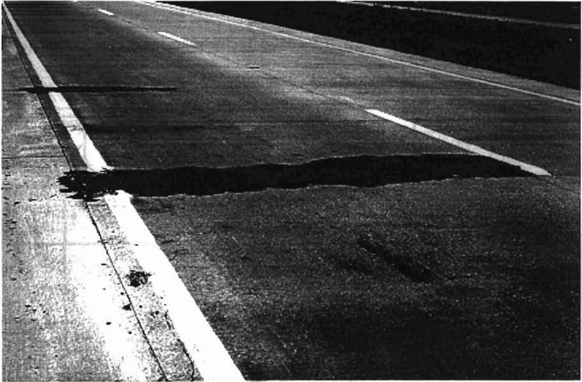
Figure A55. Patch on F-219(35) northbound.
