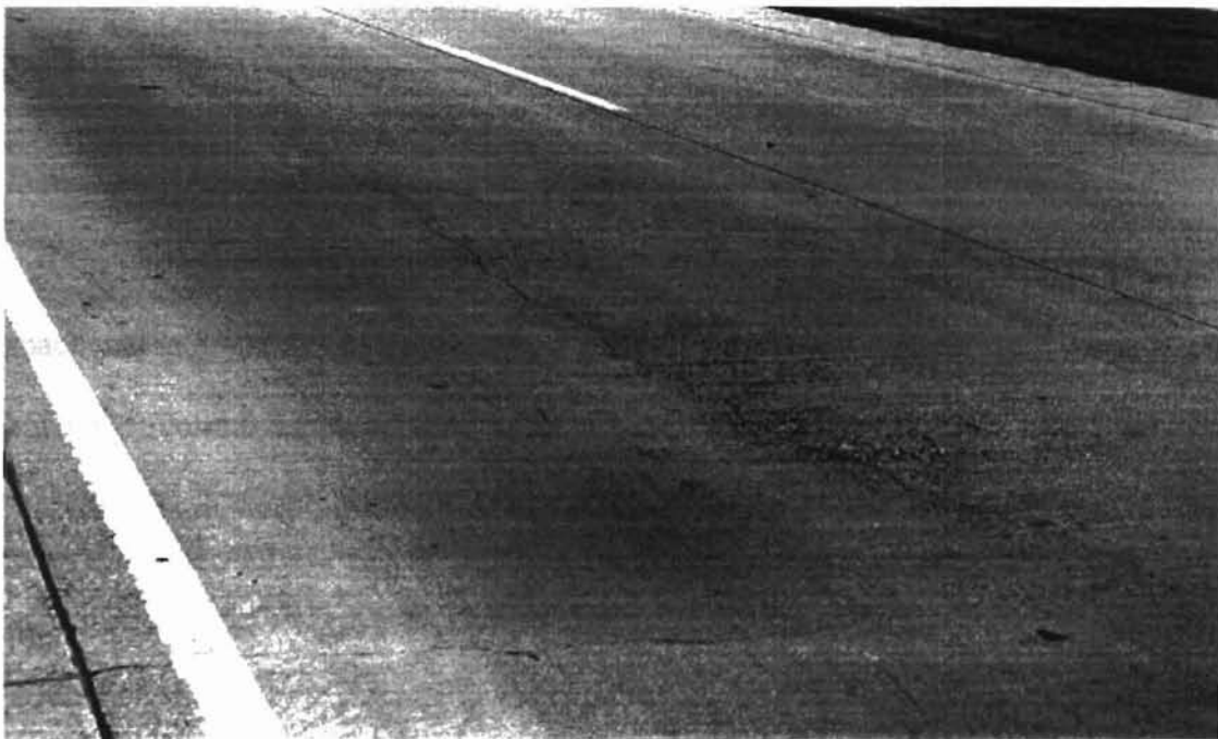
Figure A3. The longitudinal crack in MABRF-53(141)
