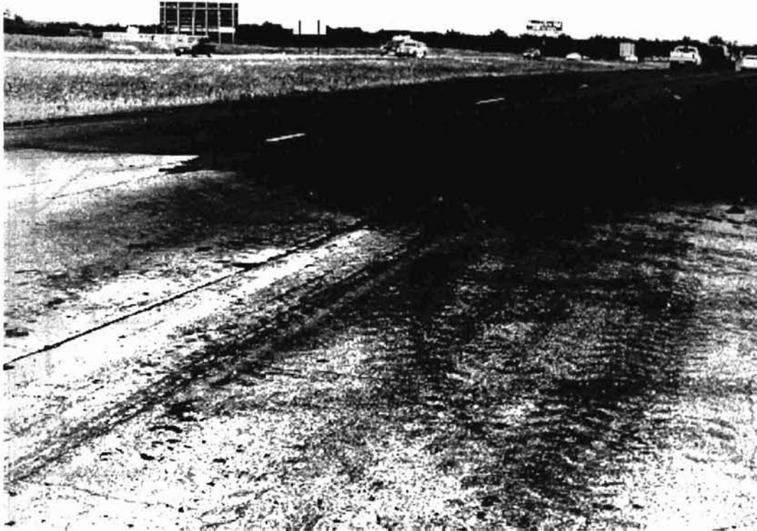
Figure A90. Asphalt overlay typical on I-35 CRCPs in Murray and Carter counties.
