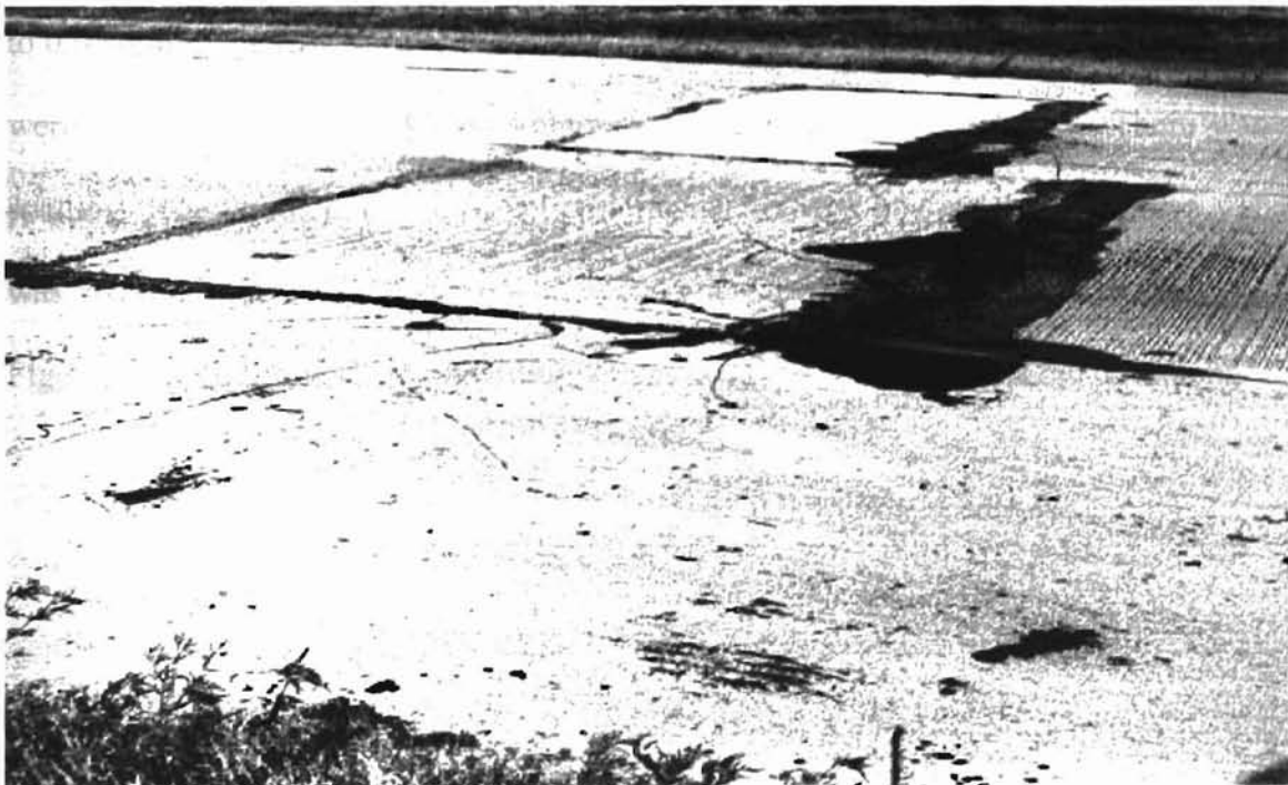
Figure A23. Patch next to repair westbound
