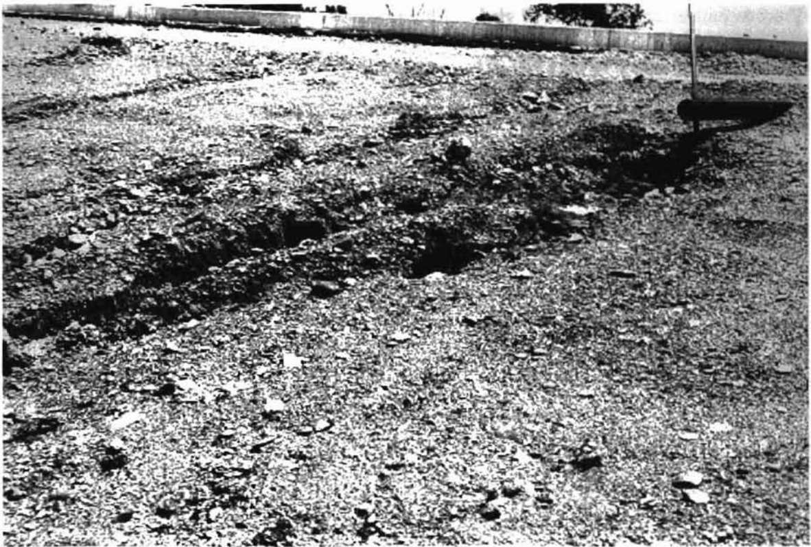
Figure A95. Outlet of drainage under pavement and erosion of embankment.
