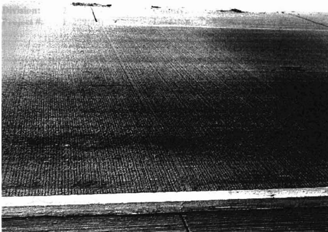
Figure A43. Typical pavement condition on MAF-186(183).
