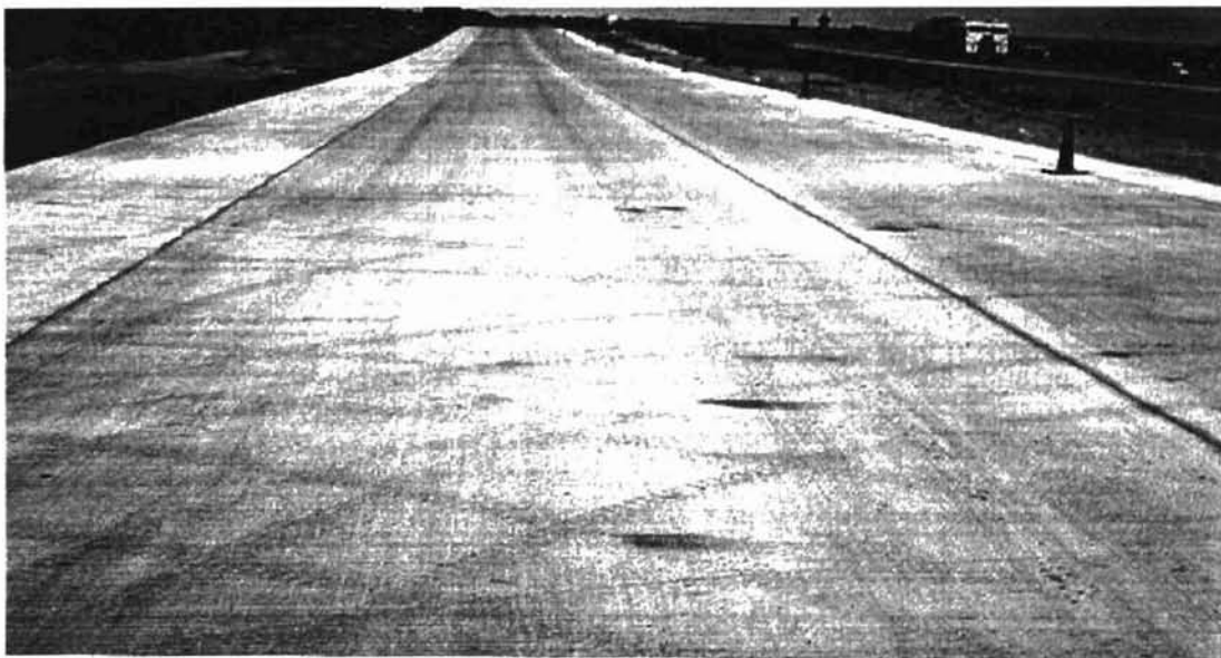
Figure A82 Westbound NH-8N(001) under construction. Traffic moving in both directions in eastbound lanes.
