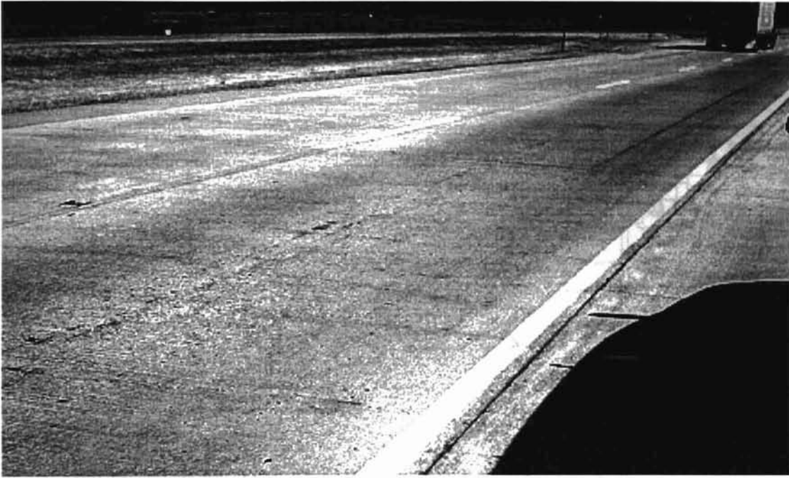
Figure A46. Typical pavement condition of F-299(45) northbound.
