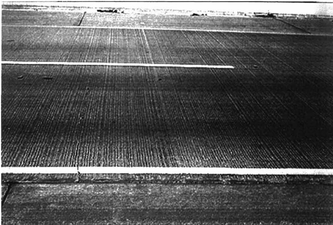
Figure A41. Typical pavement condition on MAF-186(185) southbound.
