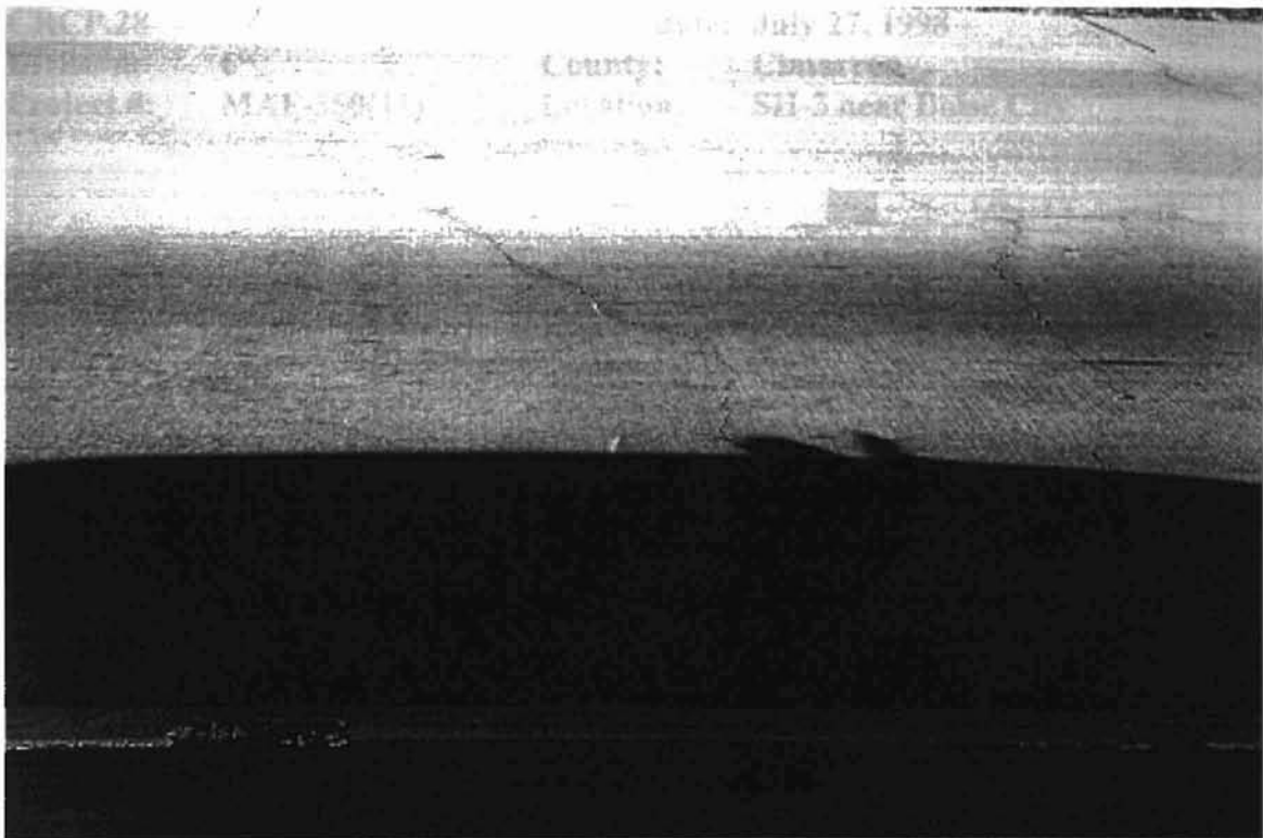
Figure A75. Curved cracks typical on IM-40-2(119) eastbound.
