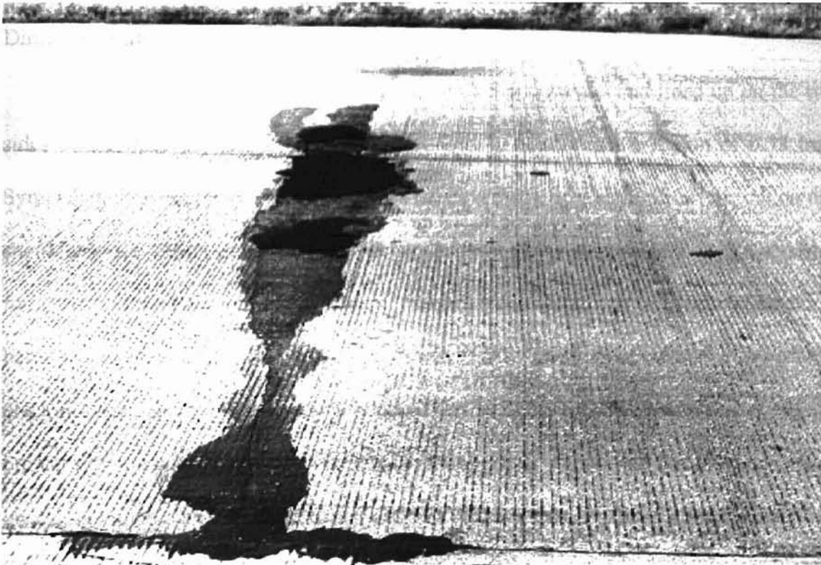
Figure A62. Patch on IR-40-5(169) westbound.
