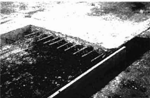
4. 450 mm (18") longitudinal reinforcement exposed.
