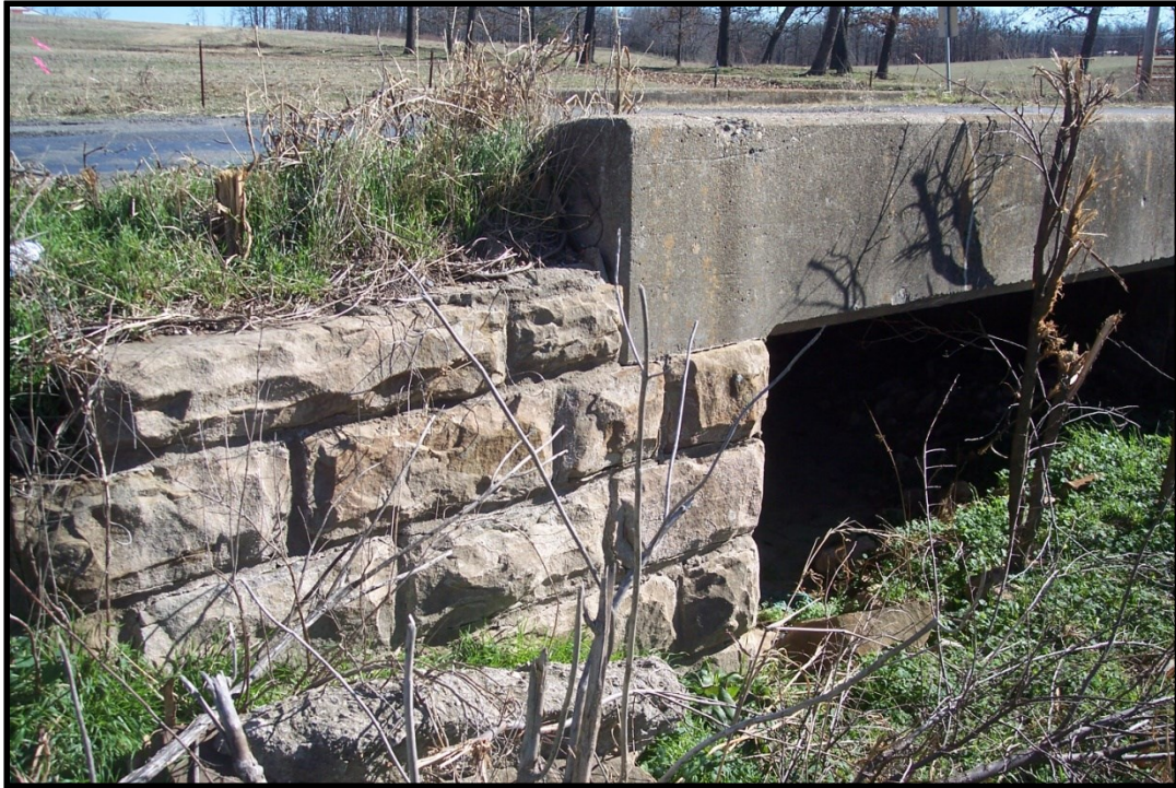
Figure 2.10. Bridge constructed in 1939 by WPA labor 0.7 miles north of Chance in northern Adair County.
