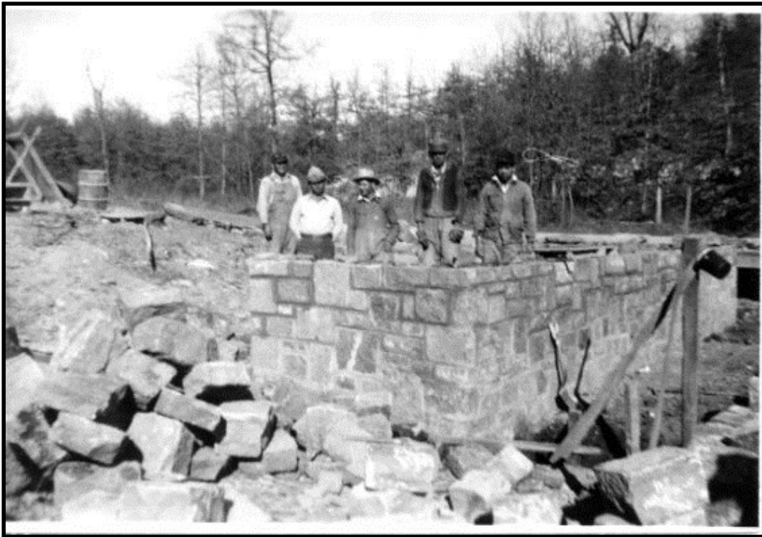
Figure 4.3. Willow Springs CCC-ID Camp enrollees constructing a bridge abutment near Willow Springs Camp Road in southern Adair County. Undated photograph.
