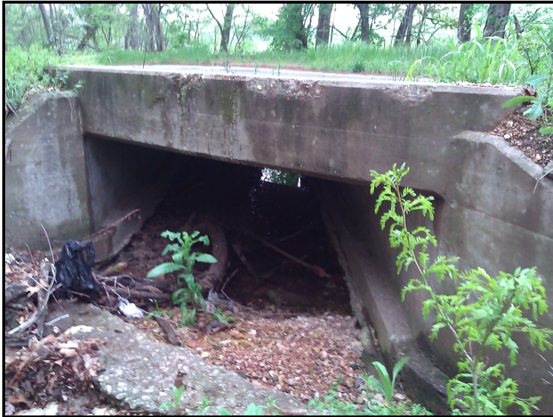
Figure 2.11. Culvert constructed in 1939 by WPA labor two miles west of Chance in northern Adair County.
