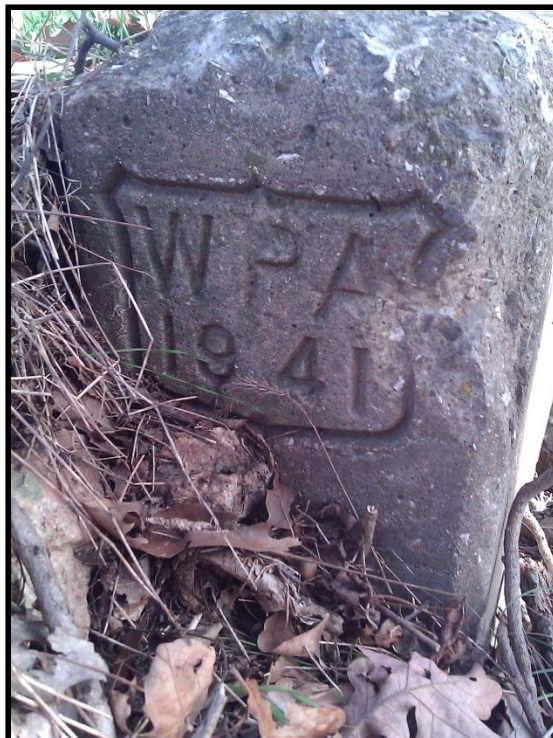
Figure 2.12. Culvert constructed in 1941 by WPA labor near Horn School in southern Adair County.
