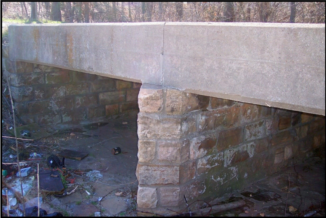
Figure 2.9. Bridge constructed in 1939 by WPA labor 1.4 miles north of Chance in northern Adair County.
