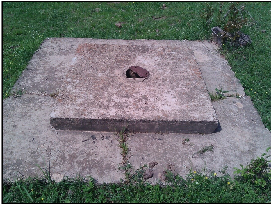
Piney School Water Well. Spring 2012.
