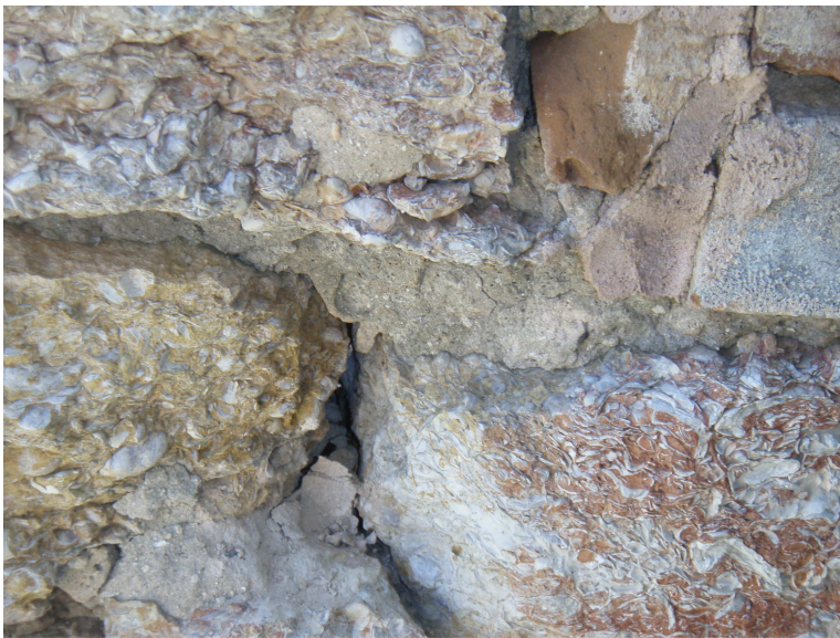
Figure 8. multi-generational mortars in stone wall at Fort Washita. Samples were restricted to 1st generation mortar behind later pointing.
