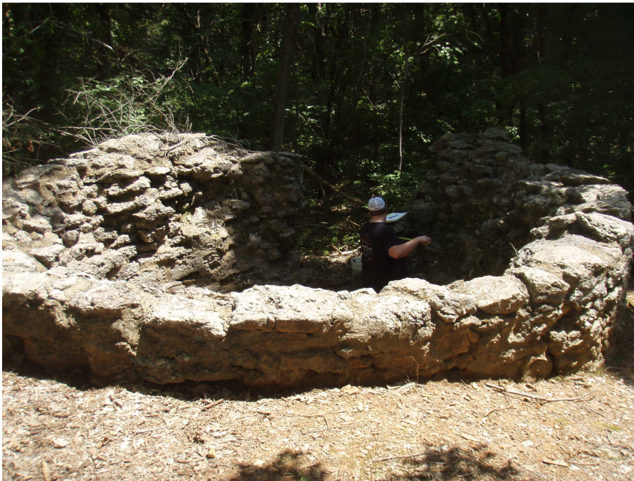
Figure 10. Top view of lime kiln at Fort Towson. This structure is mostly original, but contains some re-pointing.
