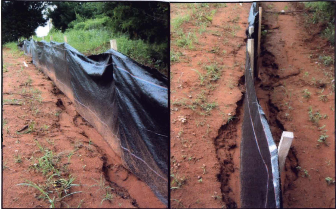
Figure 1.1: Silt fence undermined on a highway construction project near Stillwater, OK
