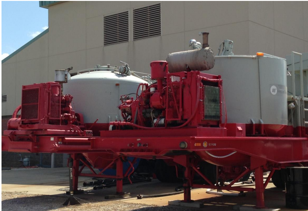
Figure 3.5: Fluid Mixing and Storage Tanks
