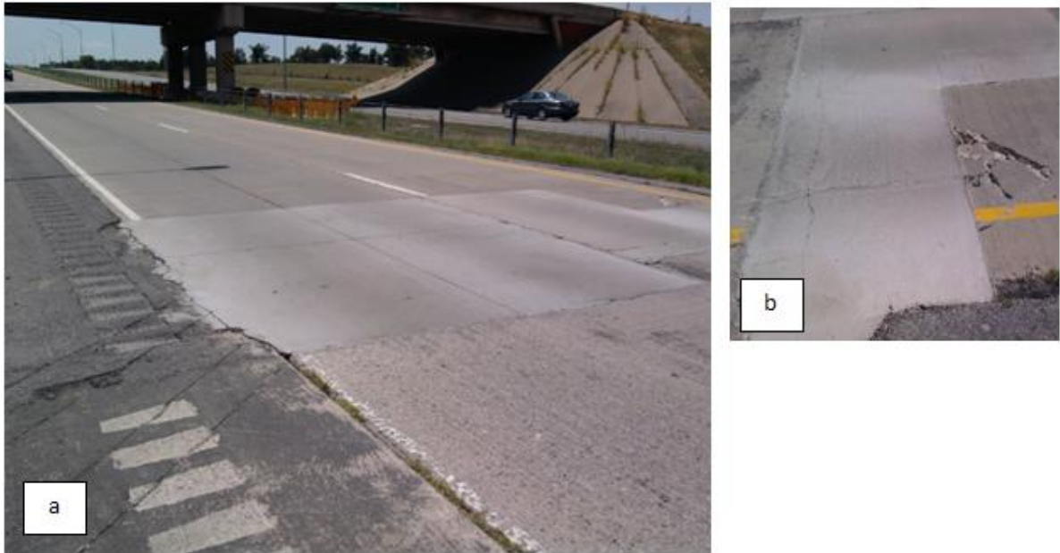
Figure 2.15 – Photo a shows the repaired panels at the north end of the overlay. Photo b shows a cracked panel at the west end of the overlay.
