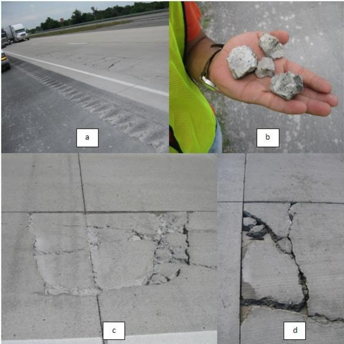
Figure 2.25 - Photos showing the failures of panels in the right wheel path of driving lane of the overlay. Photo a shows failures observed in continuous panels. Photo b shows the pieces of concrete that came from the failed panels. Photo c shows individual panel failures, typically seen at the intersections. Photo d shows drainage problems in the pavement and also the damage resulted because of it.
