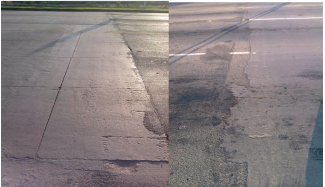
Figure 2.35 - Approach on US 177 from north showing absence in panel failures. Note the small difference in the elevation between the approach and leave pavements.
