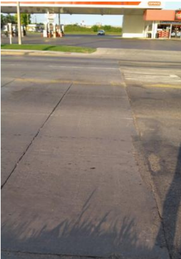
Figure 2.32 - Approach on US 177 from south on showing excellent condition of initial panels.
