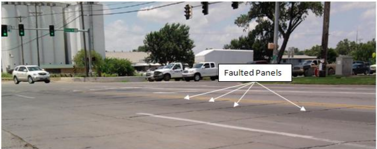
Figure 2.41 - Photo showing faulting as seen from east end of the intersection. A repetitive noise was heard from the tires of the vehicles when they passed on the faulted panels.
