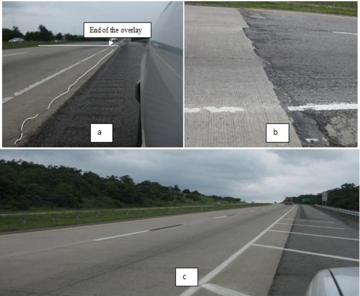
Figure 2.9 - Photo a shows the 13 panel long longitudinal crack at the end of the overlay. Photo b shows the transition of concrete into asphalt at the end of the overlay. Photo c shows overall good condition of the overlay.
