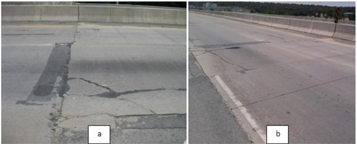
Figure 2.13 - Initial panels facing block cracking as shown in photo a. The first panel is replaced after initial failures with a full size panel as shown in photo b.
