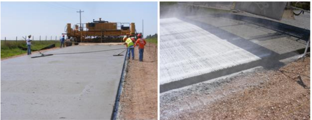
Figure 2.49 - Photos show the construction of the overlay. (Photos in Figs 2.48 & 2.49 courtesy of Chris Westlund, ODOT).
