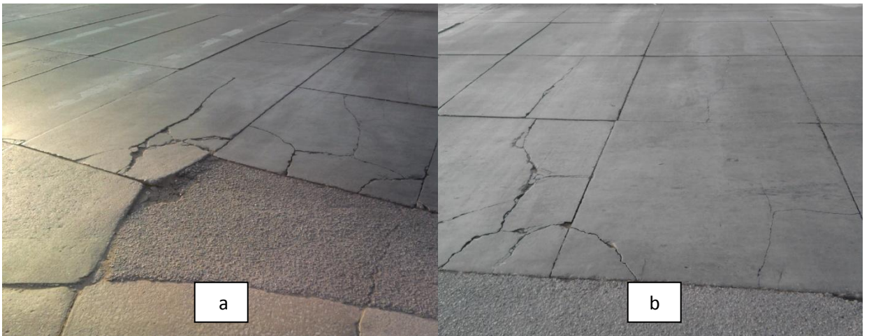
Figure 2.44 - Large block cracking at the east end of the intersection where the overlay is adjacent to the gas stations. The shadows shown in photo a show the difference in height between to the overlay and the adjacent asphalt. Additional block cracking can be seen in photo b.
