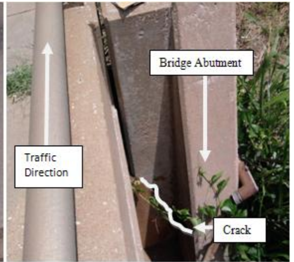
Figure 2.39 - Cracking in abutments of the bridge.
