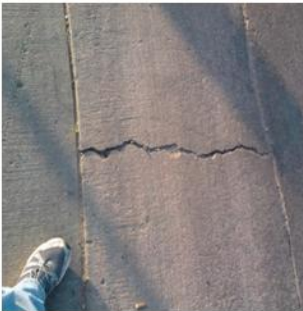
Figure 2.36 – Distress cracking in the shoulder.
