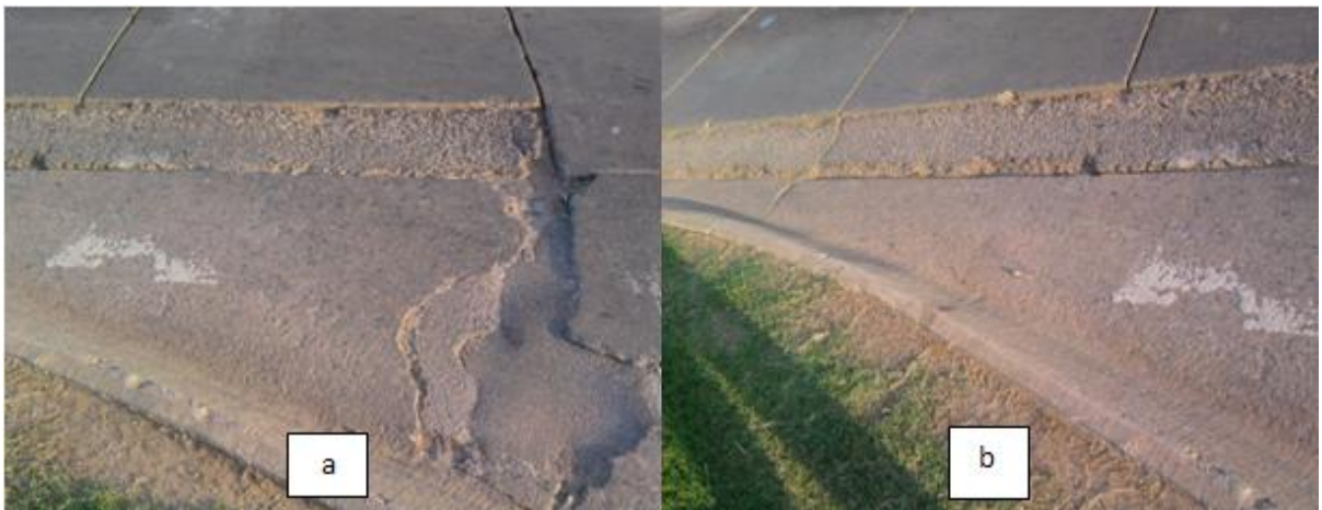
Figure 2.42 - Photos a and b showing faulting as overlay turns from west SH 51 to north US 177.
