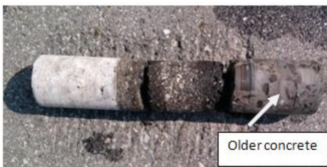
Figure 2.27 – Core from location 9.
