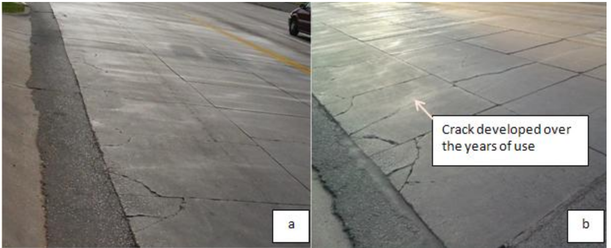
Figure 2.43 - Photos at the entrance to the gas station showing how the cracking has changed between 2004 and 2010. Photo a was taken in 2004 (David Cline, MacArthur Associated Consultants) and photo b is taken by the research team in 2010.
