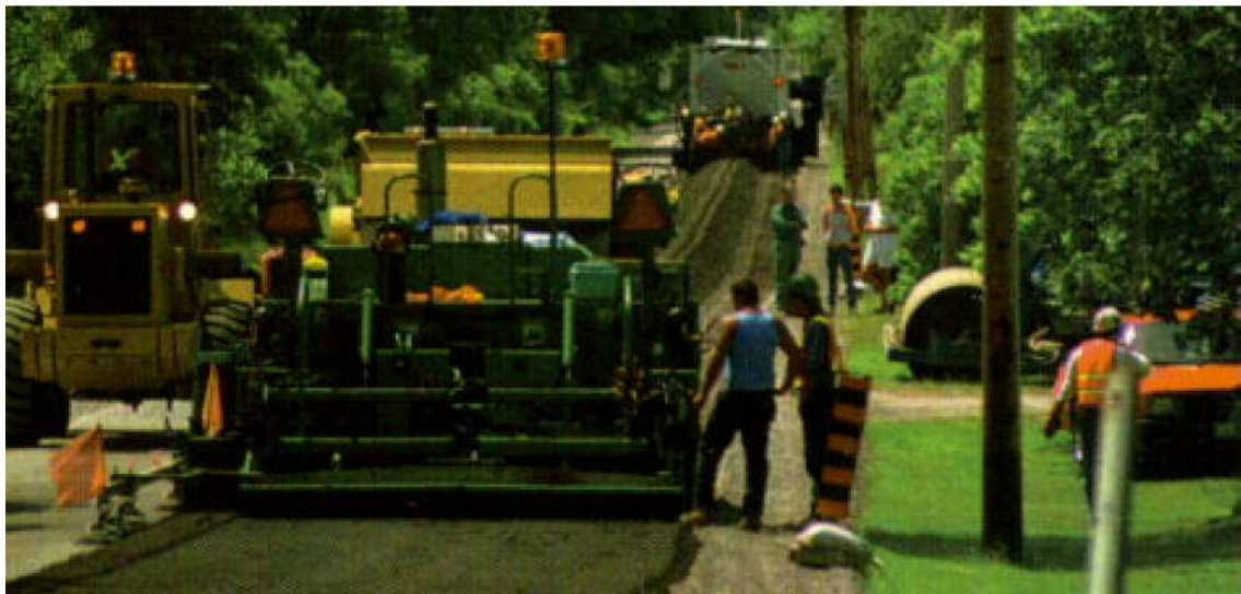
FIGURE 2-4 A Single Unit CIR Train Deposits the CIR Mixture in a Windrow [10].
