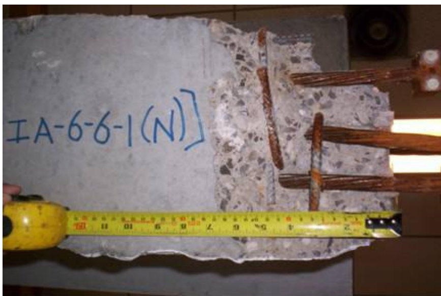
Photo showing the damage at the Bottom surface of North end of beam IA-6-6-1
