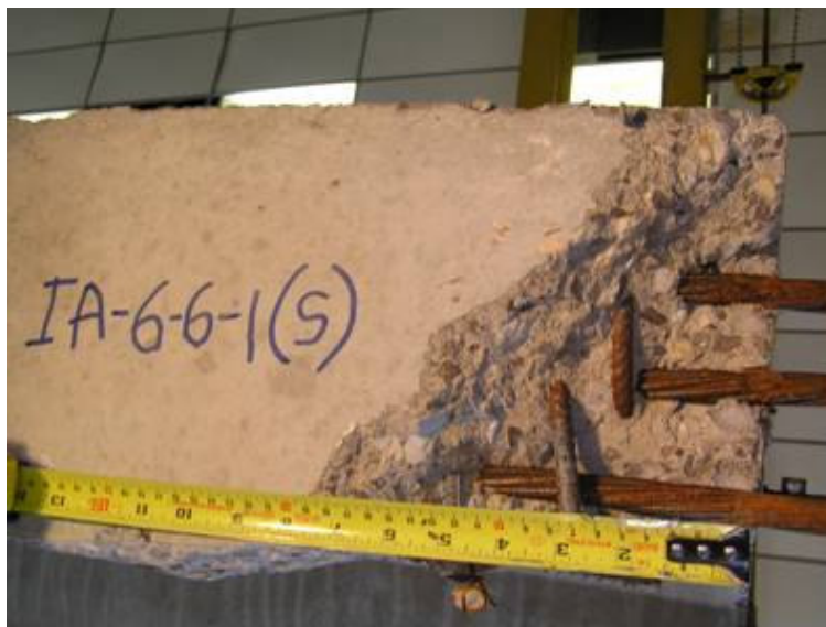
Photo showing the damage at South end caused during transportation
