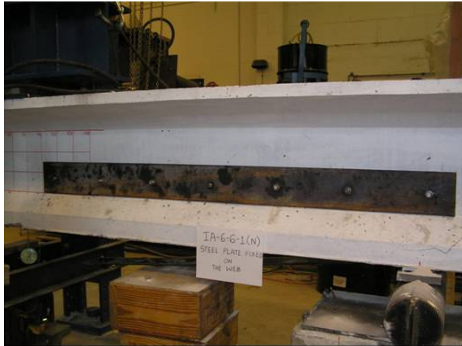
Photo showing the external steel plate attached on the web for compensating the horizontal reinforcement at the North end.
