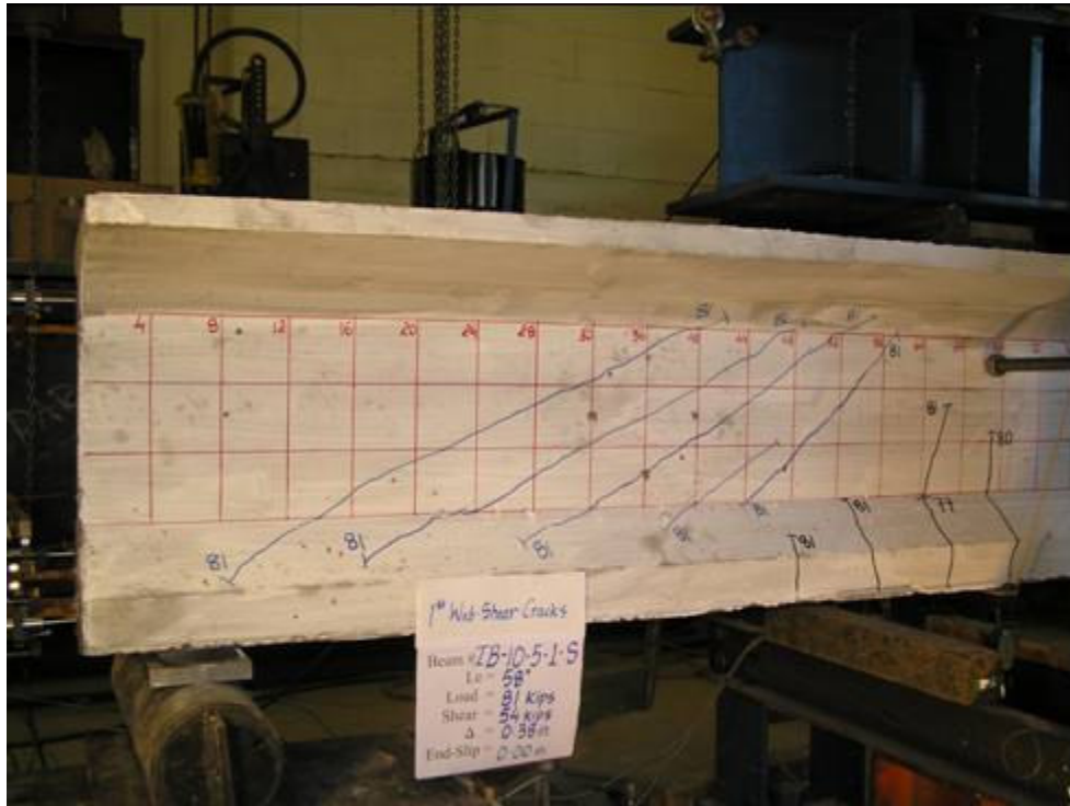
Photo of the South end of the beam IB-10-5-1 showing the first web shear cracking
