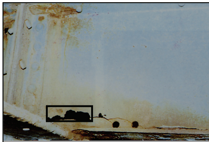
Figure 3.3: Photo of Corroded Web
