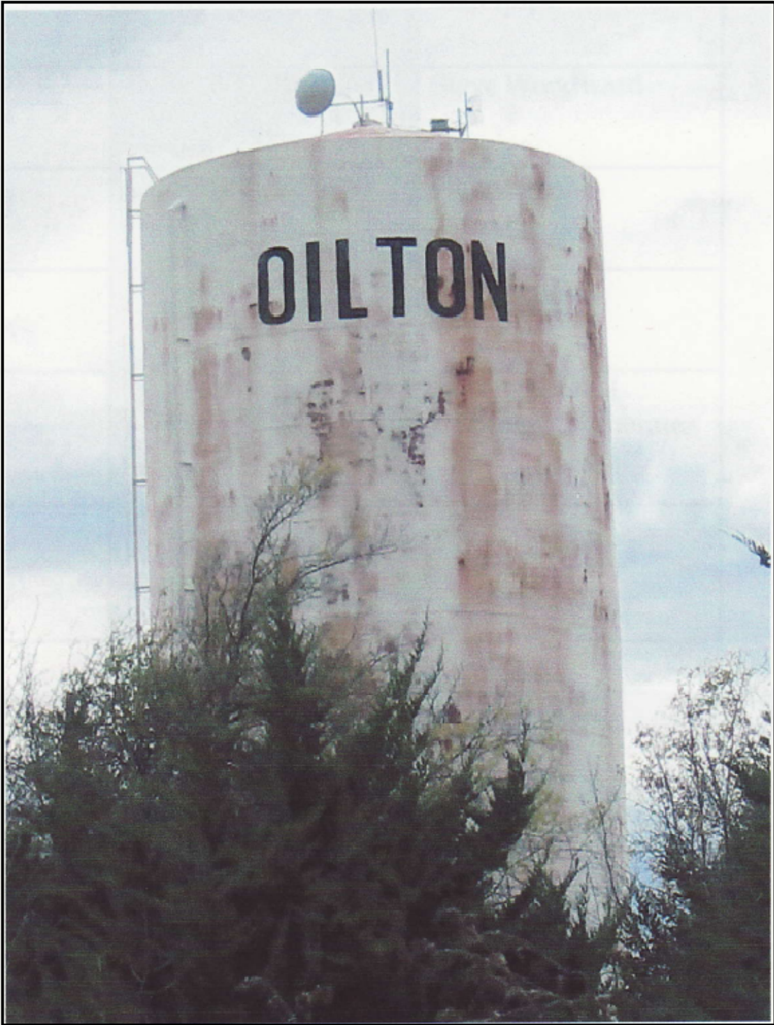
Figure 2: Picture of the 350,000 gallon Standpipe outside the town.
