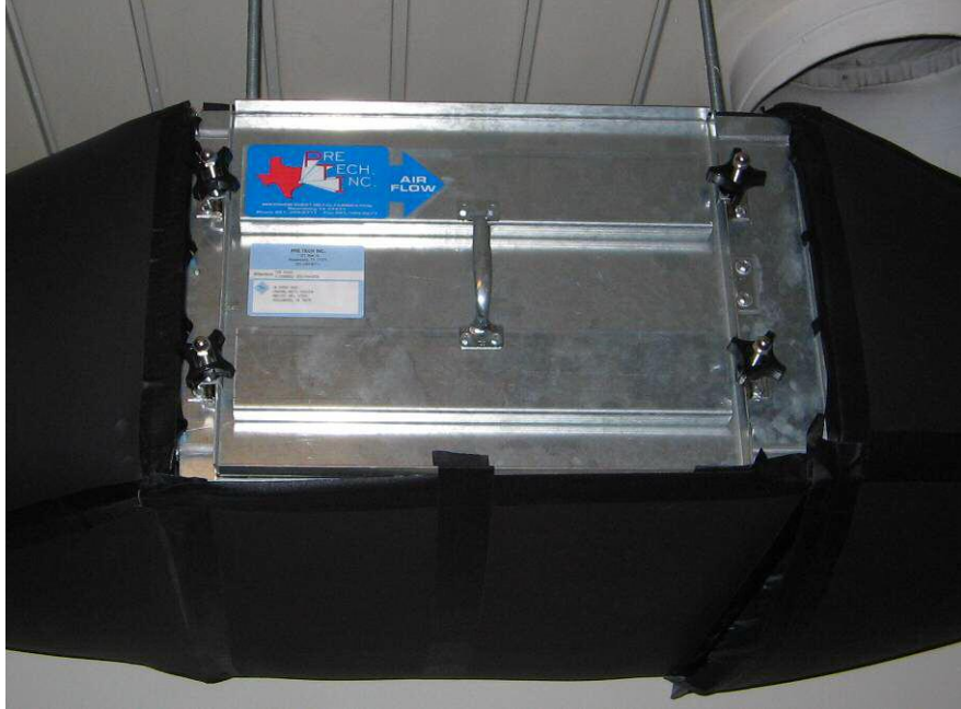
Figure D-4 Air filter housing on third level
