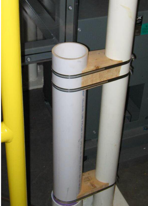
Figure D-6 Cooling coil condensate drain fill pipe
