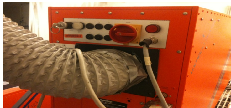
Figure 34 Laser module gas exhaust system
