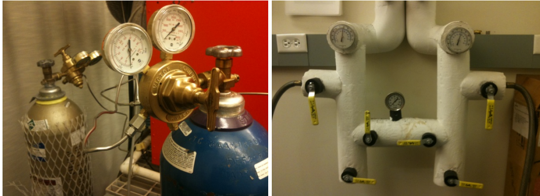
Figure 35 Gas cylinders and cooling water supply
