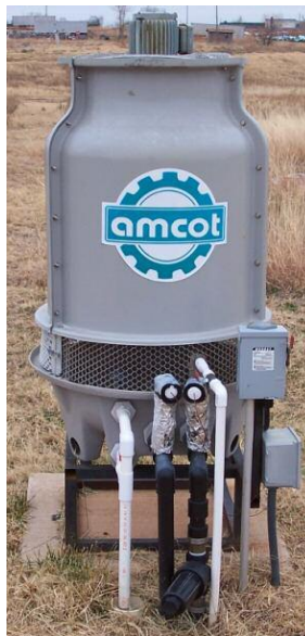
Figure 1-3. Cooling Tower [Gentry, 2007]
