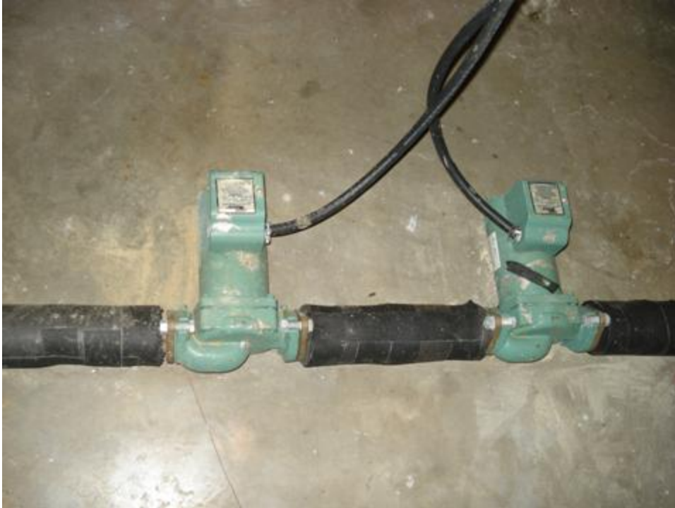
Figure 3-16. Taco pumps in series
