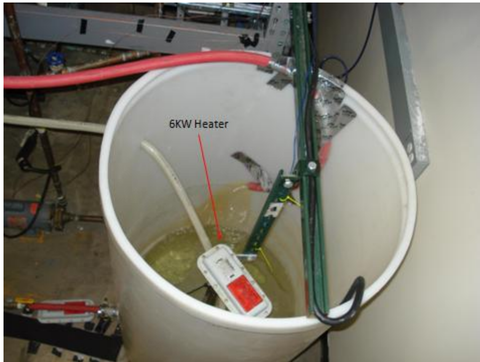
Figure 3-19. Water batch tank with customized heater
