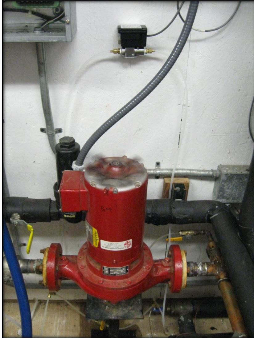
Figure 5-2 Pump and Pressure Transducer
