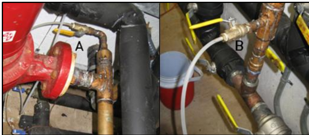
Figure 5-4 Shutoff Valves A and B at Inlet and Exit of Pump
